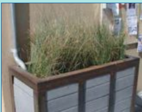
ABOVE: A downspout planter is a structure that is designed to allow stormwater from roof gutters to flow through and be used by the plants.
