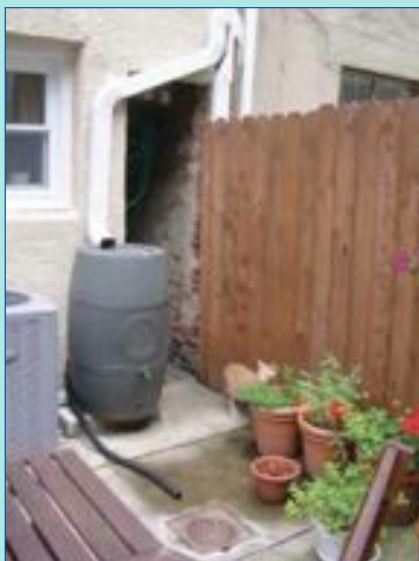
ABOVE: A rain barrel installed in the backyard of a South Philadelphia home.
