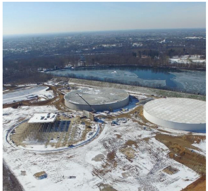
▲ Recent construction projects, such as construction of the East Park Storage Tanks, focus on replacing aging facilities to better serve our customers.
