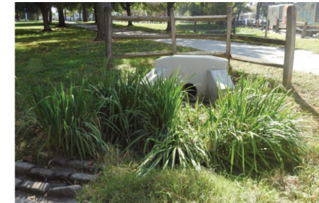
This image showcases how water enters into the rain gardens from the street (the blocks in the lower left), as well as how smaller rain gardens are connected to larger rain gardens via a pipe network (under the sidewalk).
