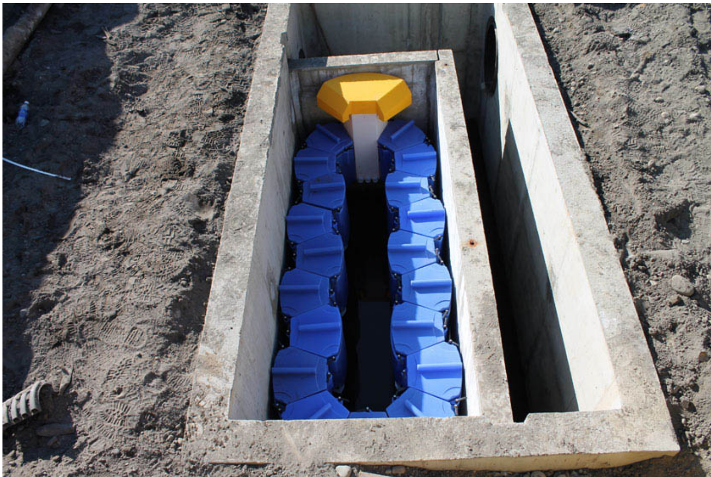
An example of a media filter installation in Philadelphia
