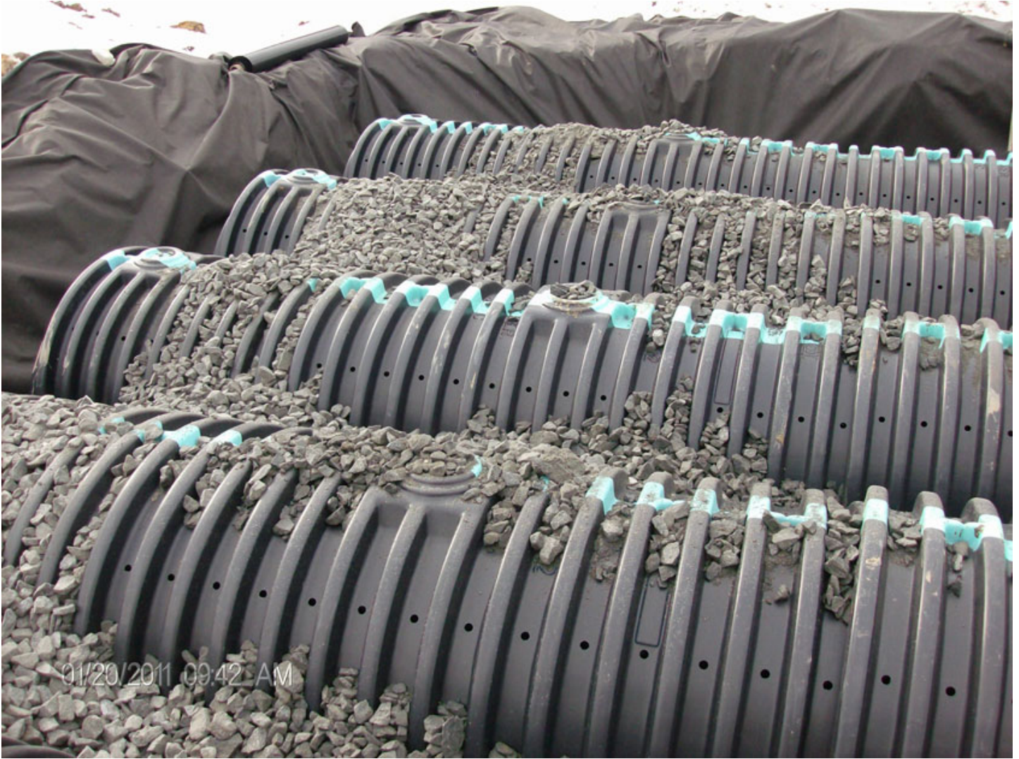
A subsurface detention basin represents one of the Philadelphia Water Department's least preferred SMPs.
