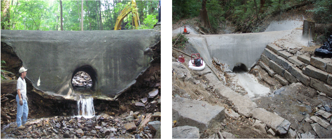
Figure 3-101: Upstream view of WScul116 pre-construction (left); Downstream view of WScul116 post-construction (right).
