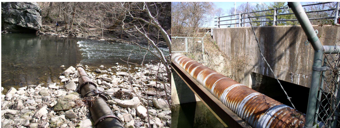
Figure 2-16: Example of a pipe assessed in infrastructure trackdown.
