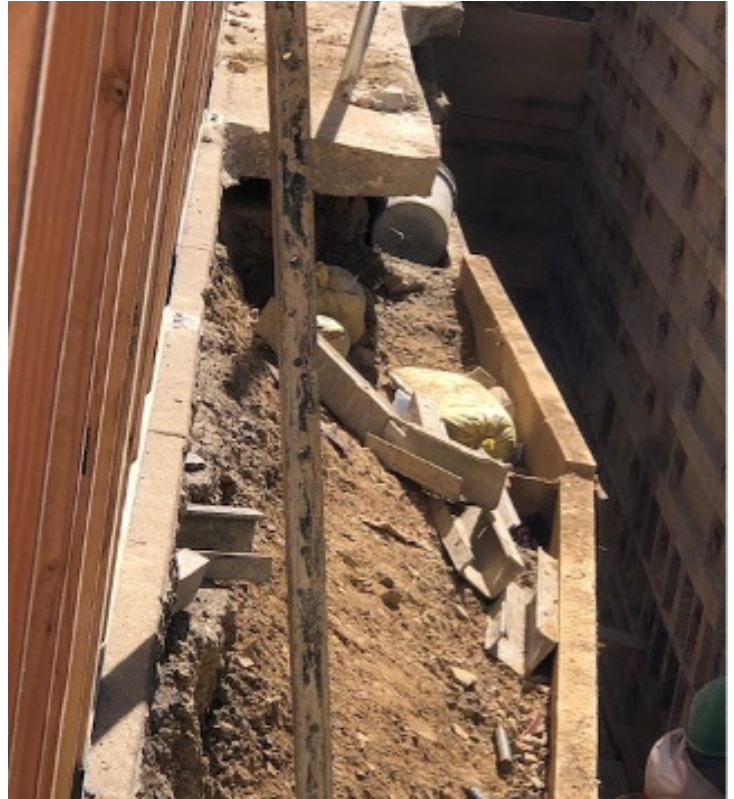
Above: On-site excavation without proper shoring puts water mains at risk.
