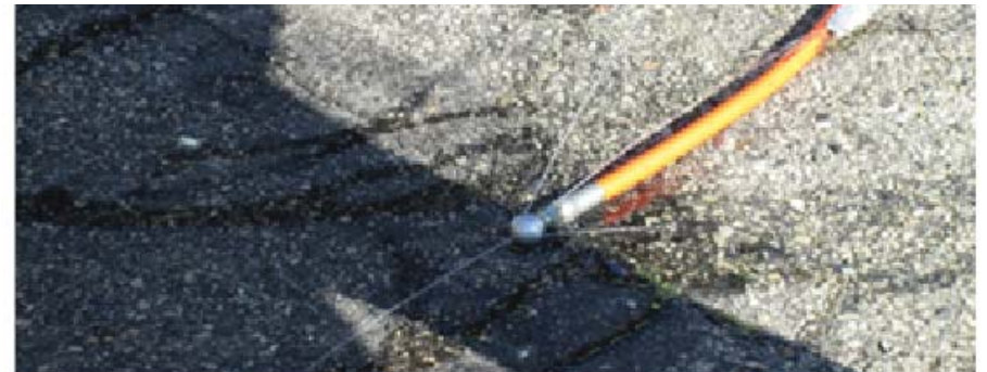
Figure 3-3. Small penetrating nozzle with one front facing and six rear-facing jets
