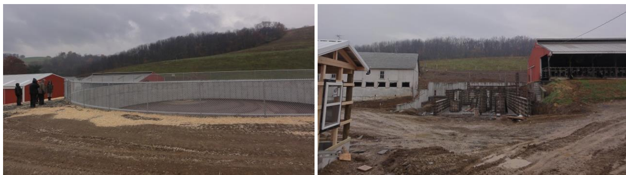
Figure 5-12: Durkin Farm Headquarters (a) Completed Liquid Manure Storage Basin (November 2016) (b) Dry Manure Storage Basin Under Construction (November 2016)
