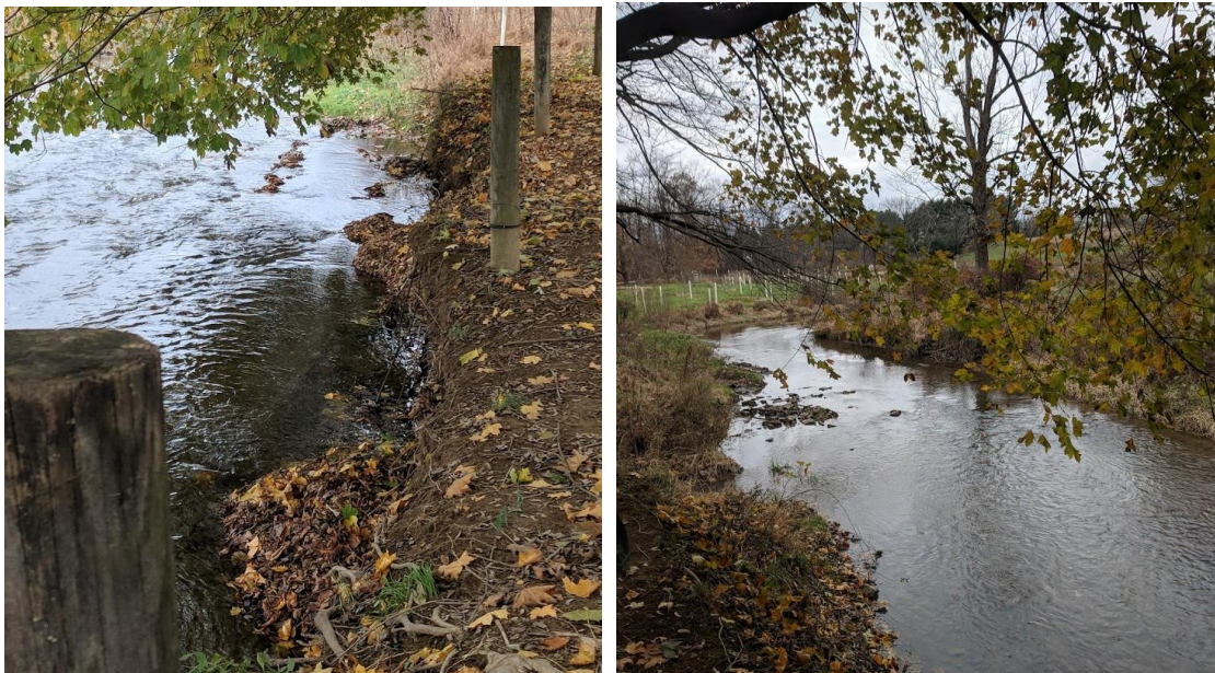
Figure 5-6: Irish Creek Streambank Erosion - (a) Right Stream Bank (b) Upstream View of the Left Bank where Stormwater Drains into the Creek
