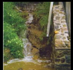
STORMWATER DAMAGE, EROSION, AND FLOODING
