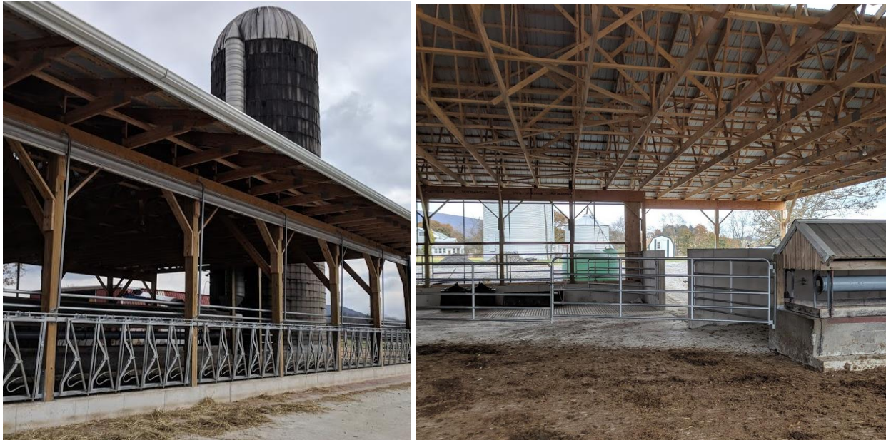
Figure 5-9: Zettlemyer Farm (November 2017) (a) Roof extends over feeding area (b) New roof from the inside of the barn, cement wall to hold dry manure
