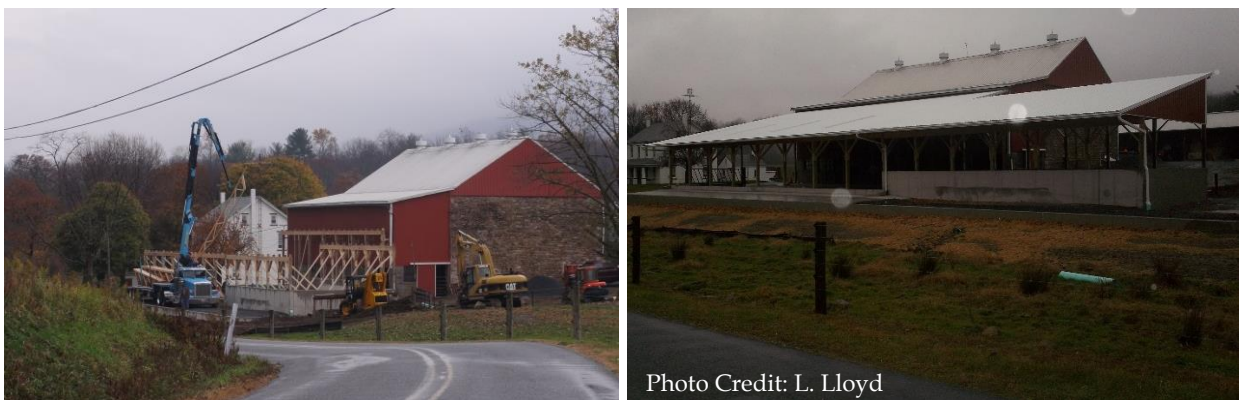
Figure 5-10: Zettlemyer, Second Farm (a) Heifer Barn Under Construction in Early November 2016 (b) Heifer Barn Improvements Completed in Late November 2016
