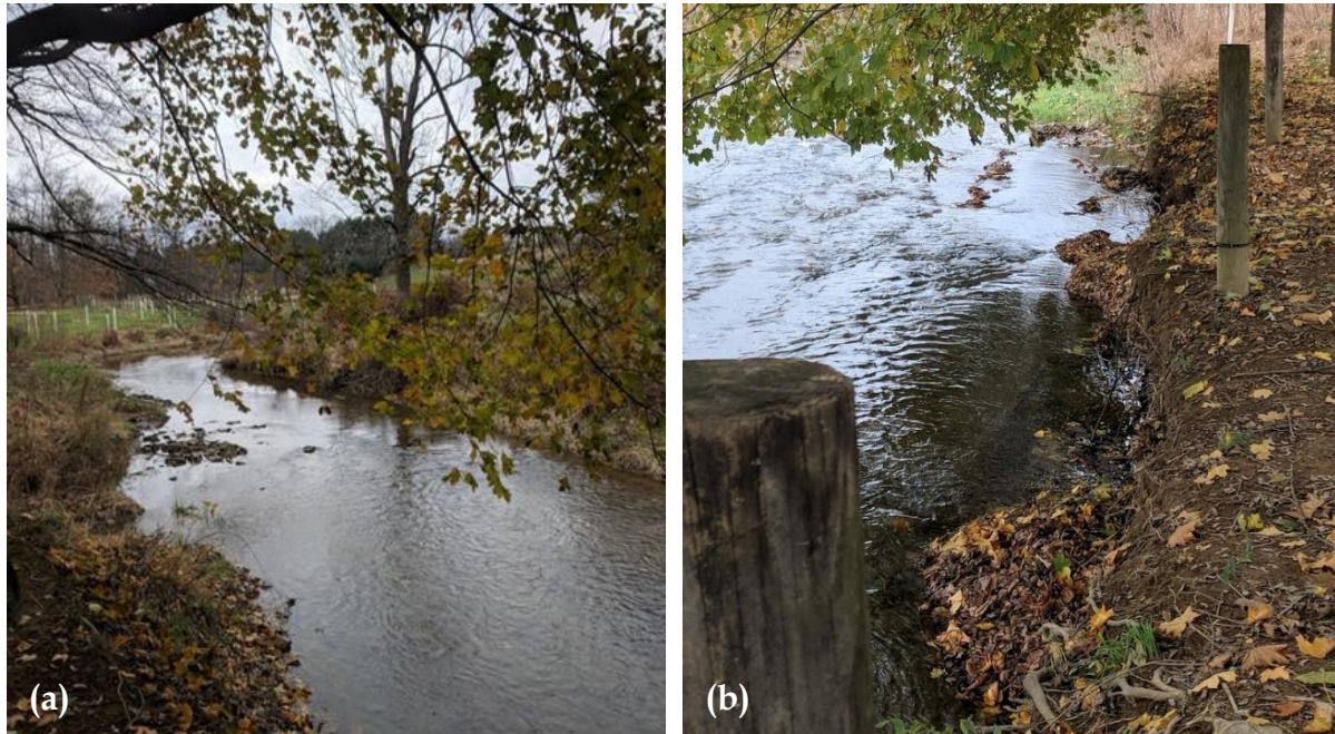
Figure 4-21: Irish Creek Streambank Erosion - (a) Upstream View of the Left Bank where Stormwater Drains into the Creek (b) Right Stream Bank
