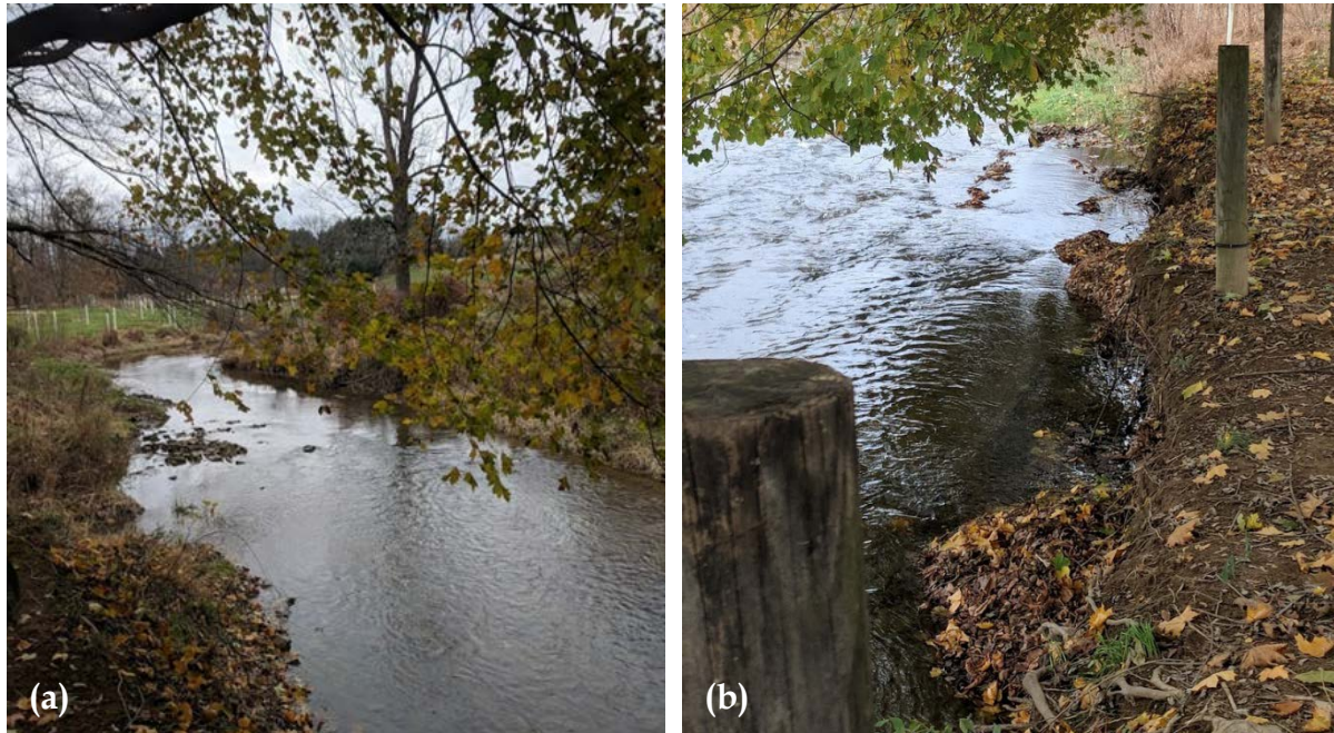
Figure 4-25: Irish Creek Streambank Erosion - (a) Upstream View of the Left Bank where Stormwater Drains into the Creek (b) Right Stream Bank
