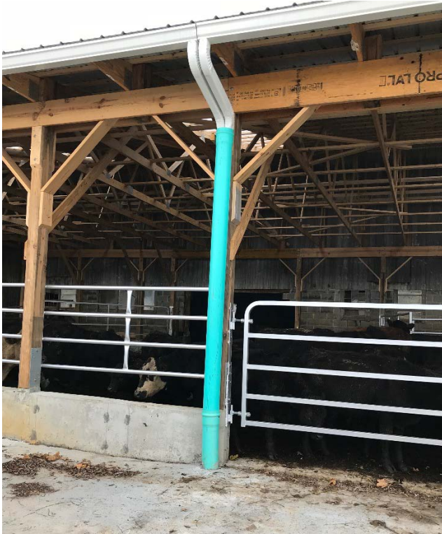
Figure 4-17: Manure Storage Area Rain Gutters at A. Burkholder Farm (November 2018)
