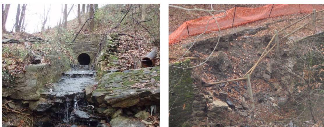
Figure 3-34: Degraded section of WScha280 (left). Degraded section of WScha142 (right).
