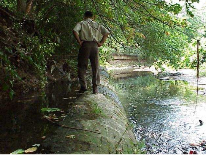
Photo 3 - Exposed Sewer Line
