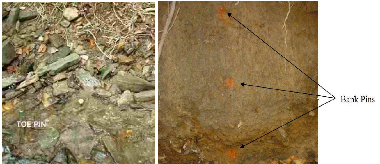
Figure 2-6: Example of Toe Pin (left) and Bank Pin (right) Setup along stream bank
