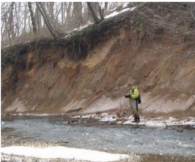
Figure 1. Eroded stream bank at Poquessing Creek
