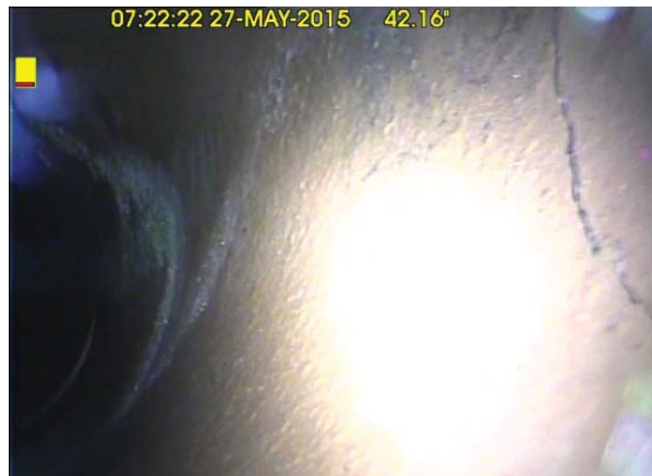
Figure 3-13. Circumferential Fracture, a Break Line that is Visibly Open and a Gap Can be Seen. The Sections of Pipe Wall are Still in Place and Cannot Move.
