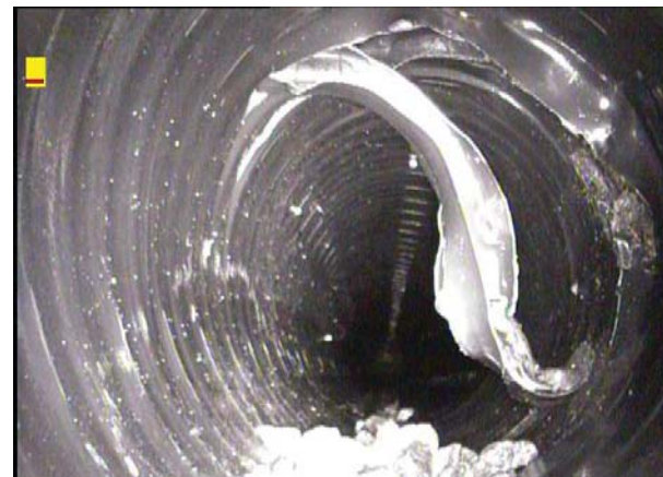
Figure 3-15. Hole, a Defect Where Pipe Material is Completely Dislodged from Pipe Wall and the Surrounding Media is Exposed.
