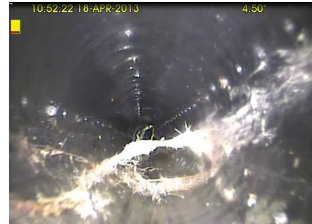
Figure 3-22. Roots - Medium: Roots that have Formed a Mass and Restrict the Flow of Water. Cross-sectional Area Lost is Greater than or Equal to 5% up to or Less than or Equal to 50% (5-50%).
