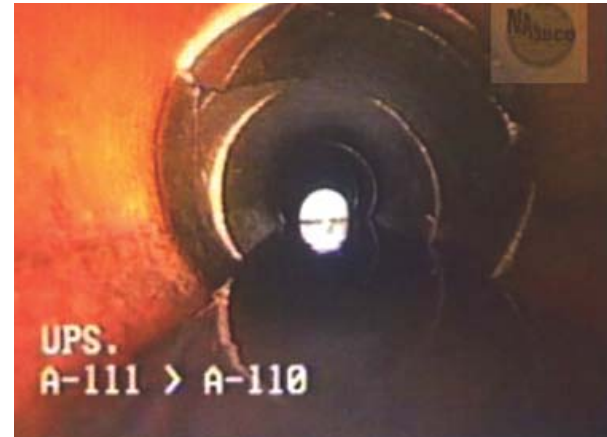
Figure 3-14. Break, a Defect Where Pieces are Noticeably Displaced and Have Moved from Original Position at Least \frac{1}{2} the Thickness of the Pipe.
