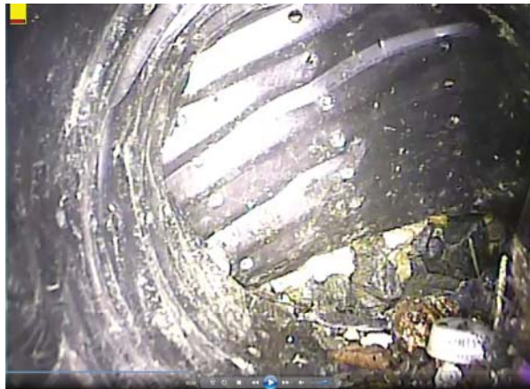
Figure 3-17. Collapse, Deformation so Great that there has been a Complete Loss of the Structural Integrity of the Pipe with More than 40% of Cross-sectional Area Lost.
