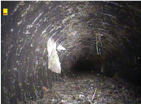
Figure 3-19. Deposited Material in the Invert of the Pipe.
