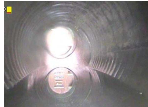
Figure 3-25. Water Level: the Depth of Water at the Observed Point in the Pipe (Includes Flowing and Stagnant Water). Water Level Sag Occurs when the Grade of the Pipe is Poor.
