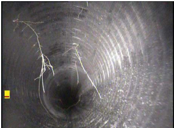
Figure 3-20. Roots - Fine: Small Diameter and Small Quantities of Roots that are Insufficient to Cause a Quantifiable Reduction of Pipe Cross-sectional Area (<5% loss).
