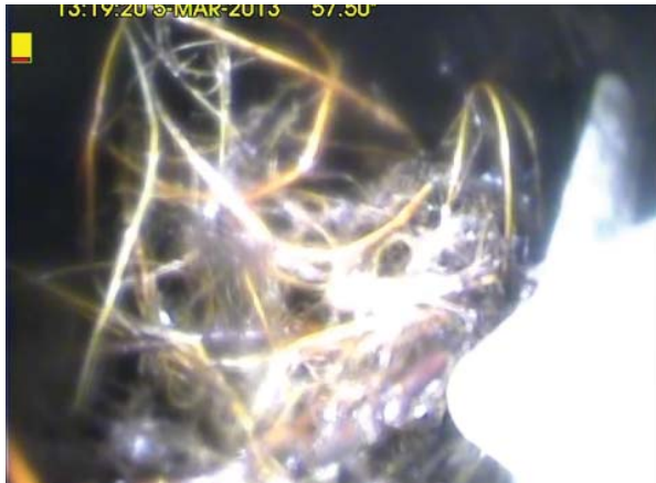
Figure 3-23. Root - Ball: Roots that have Formed a Mass, Typically in the Form of a Ball, and have the Potential to Severely Restrict the Flow. The Cross-sectional Area is Greater than 50%.
