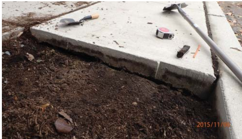
Figure 2-5. Example of Settling in a Tree Pit
