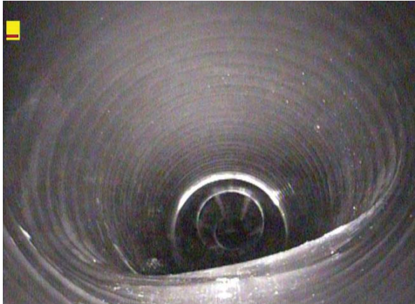
Figure 3-16. Deformation, Pipe Damage Where the Original Cross-section or Geometry of the Pipe has Noticeably Changed.
