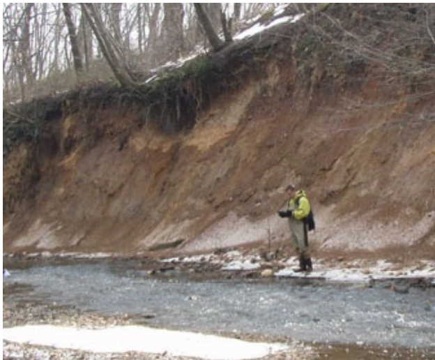
Figure 1. Eroded stream bank at Poquessing Creek NPDES Permit Nos. PA0054712, PA0026689, PA0026662, PA0026671
