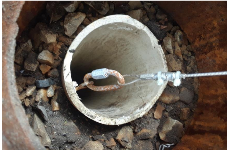
Figure 5-4 – Sensor and stainless-steel cable attachment
