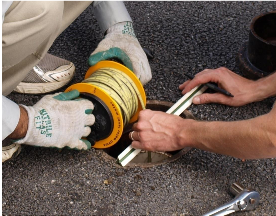
Figure 5-10 – Observation Well Depth-to-Water Measurement
