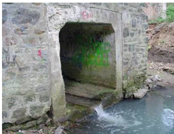
Figure 1-3 Point 99 – View from the Ground; Gorgas Run (Near the Intersection of Valley and Henry Ave)
