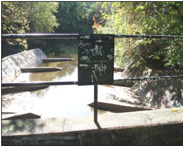
Figure 2-13 Missing CSO Notification Sign
