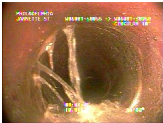
Figure 2-11: Example 5-Rating Infiltration Gusher
