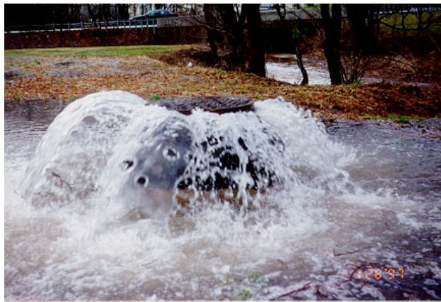
Figure 1.4.6-4 Overflowing Manhole Nearby a Stream
