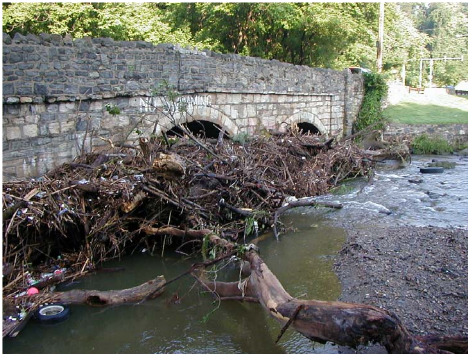
Figure 4-47 Adams Avenue after August 1, 2004 Storm
