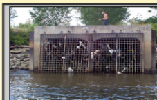
#8 D5 416 MG/yr. Delaware River Magee Street southeast of Milnor Street Twin outfall 11' x 9'
