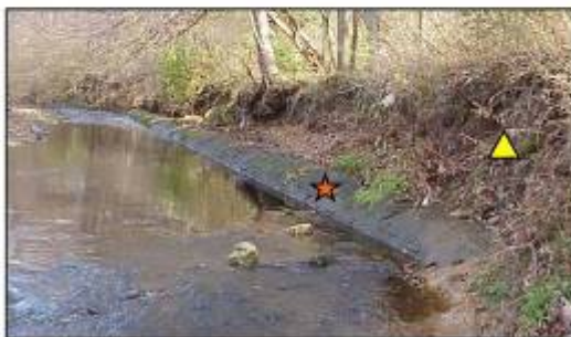
The creek at Marshall Road suffered from severely eroded banks ( triangle ) and exposed infrastructure ( star ).
