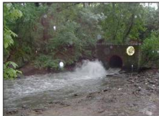
Combined Sewer Overflow at Crescentville in Philadelphia
