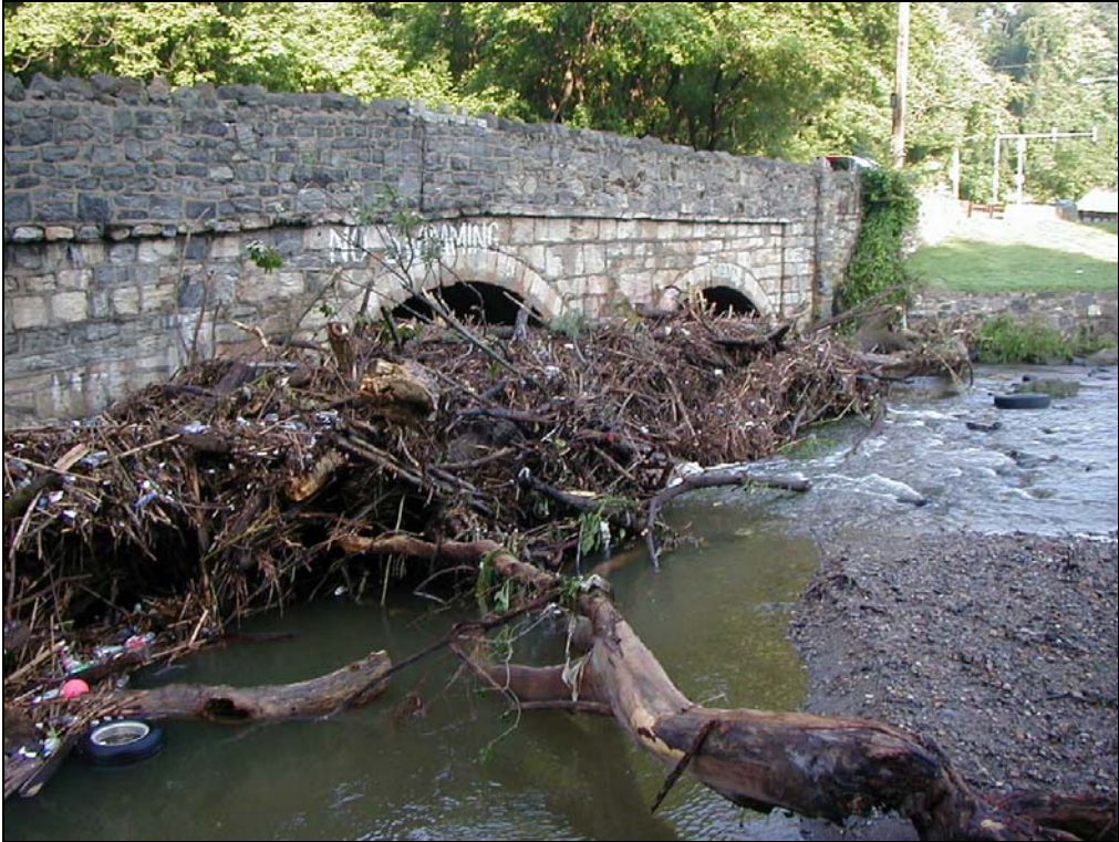
Figure 4.46 Adams Avenue after August 1, 2004 Storm
