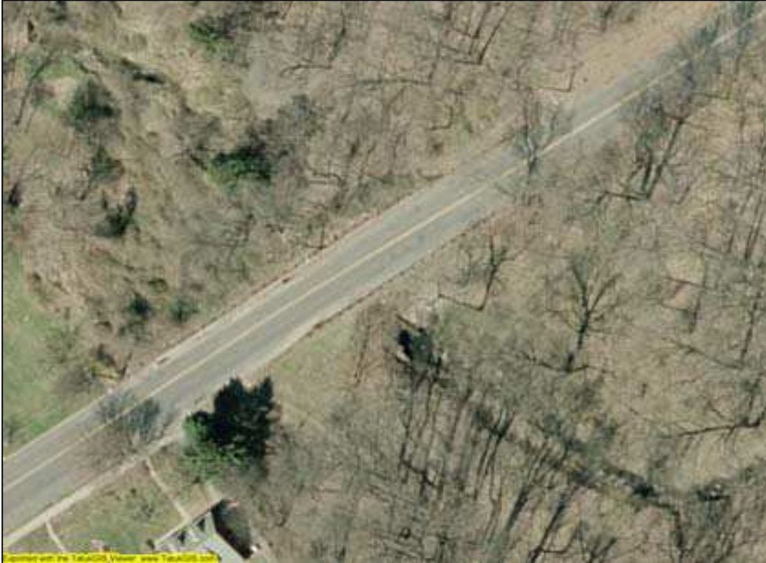
Figure 6-2 Severe Erosion Downstream of Summit Ave, Wise's Mill Run
