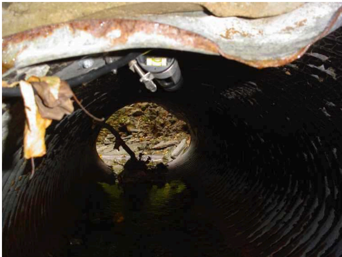
Figure J-8 Ultrasonic Down-looking Acoustic Water Level Sensor Installed in a Pipe in Cathedral Run Tributary
