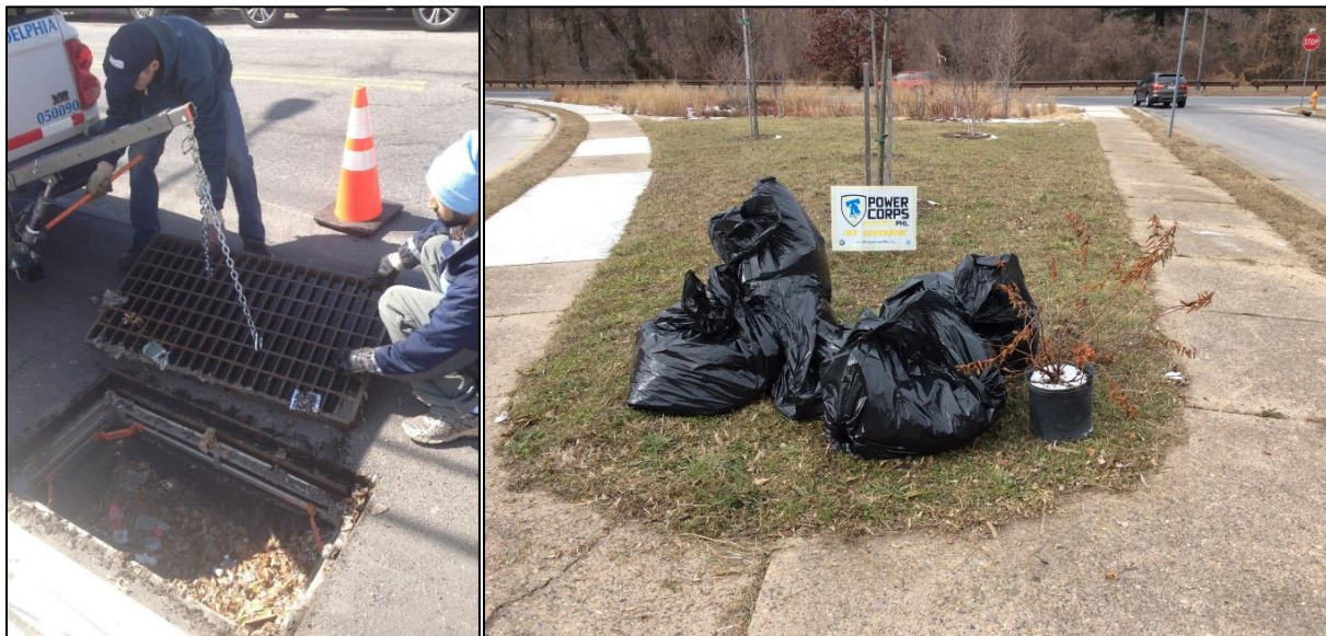
Figure 5-5: Tree trench inlet pretreatment device cleaning (left) and resulting volume of material removed from a rain garden (right) during example surface maintenance activities (source: The PWD)
