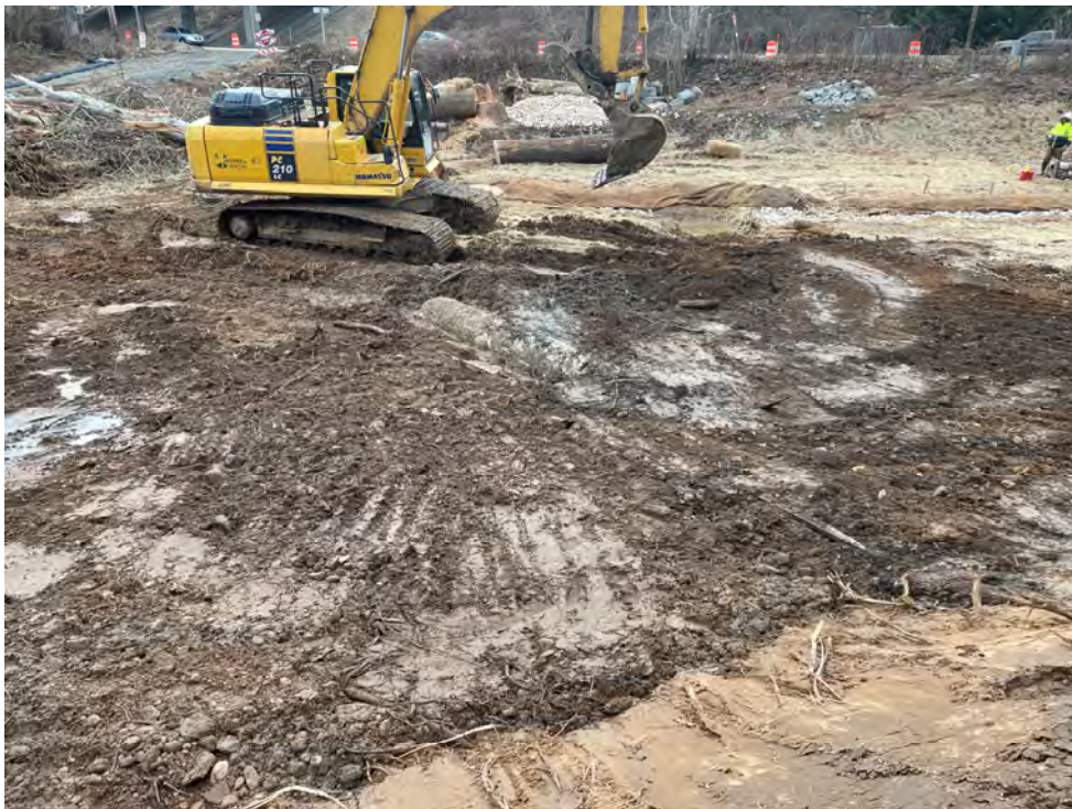
Photograph 2: Floodplain log sill during construction at UNT to Patapsco River, Baltimore County, MD. Source: JMT.
