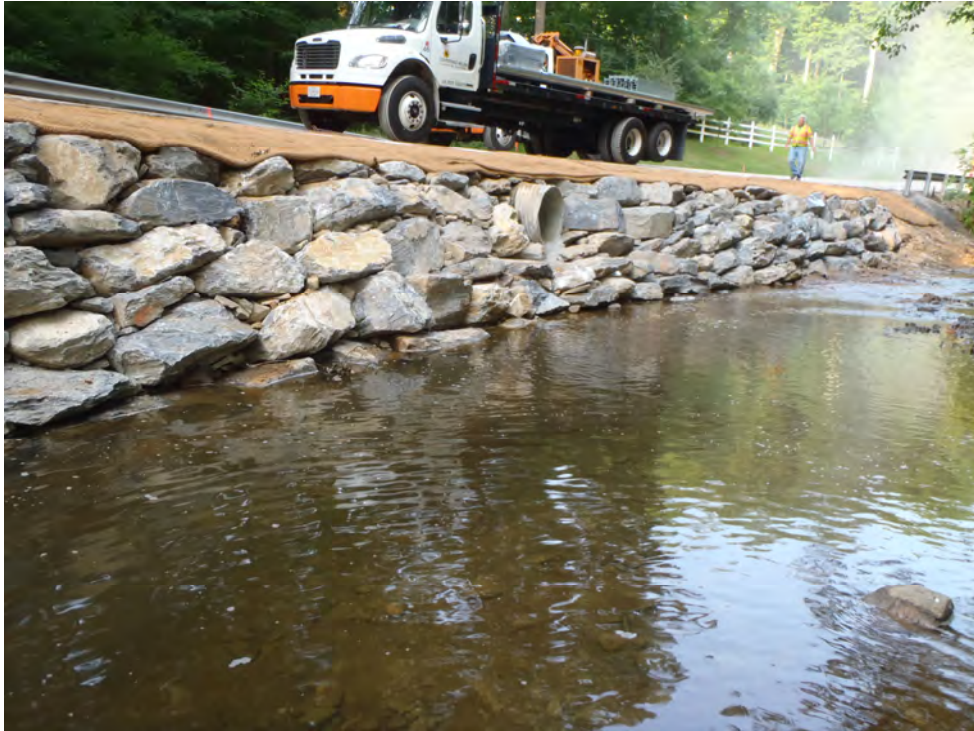
Photograph 3: Boulder wall following construction at UNT Middle Patuxent River, Howard County, MD. Source: JMT.
