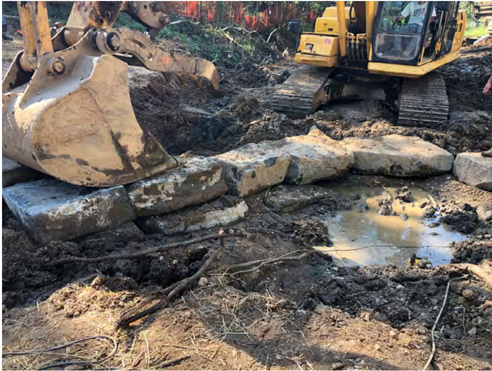
Photograph 1: Cross rock vane during construction at UNT to Patapsco River, Baltimore County, MD. Source: JMT.
