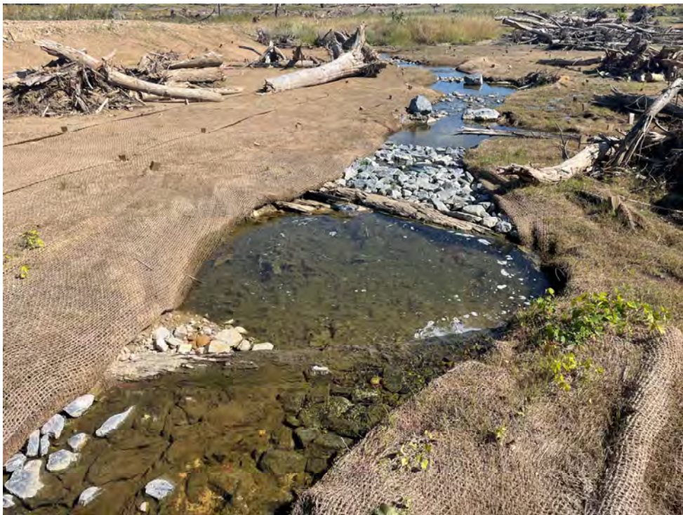
Photograph 2: Rock and roll logs following construction at UNT to Jones Falls, Baltimore County, MD. Source: JMT.
