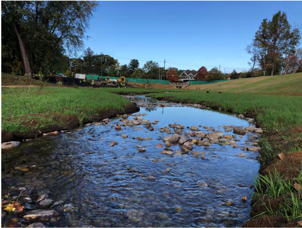
Photograph 1: Typical riffle cross section following construction at Stickney Creek, Cuyahoga County, OH. Source: JMT.
