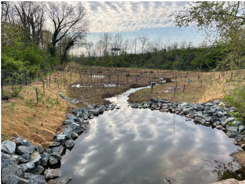
Photograph 2: Preformed scour hole following construction at UNT to Patapsco River, Baltimore County, MD. Source: JMT.
