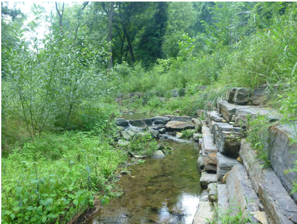
Photograph 2: Rock step pool with boulder toe revetment following construction at West Branch Indian Creek, Philadelphia, PA. Source: PWD.
