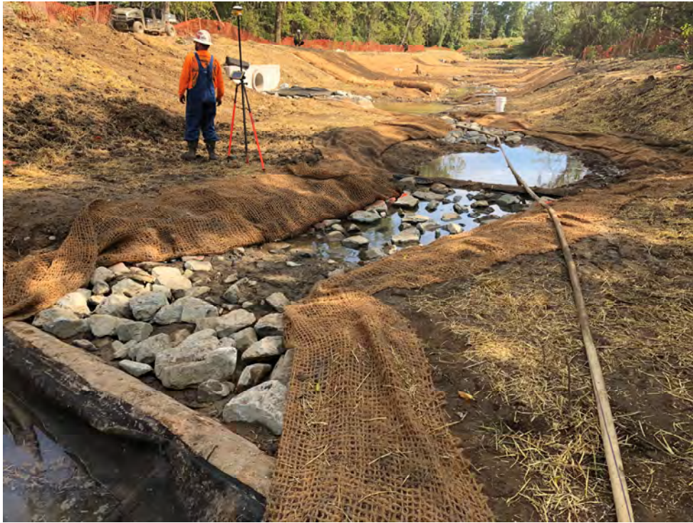
Photograph 1: In-stream log sill during construction at UNT to Patapsco River, Baltimore County, MD. Source: JMT.
