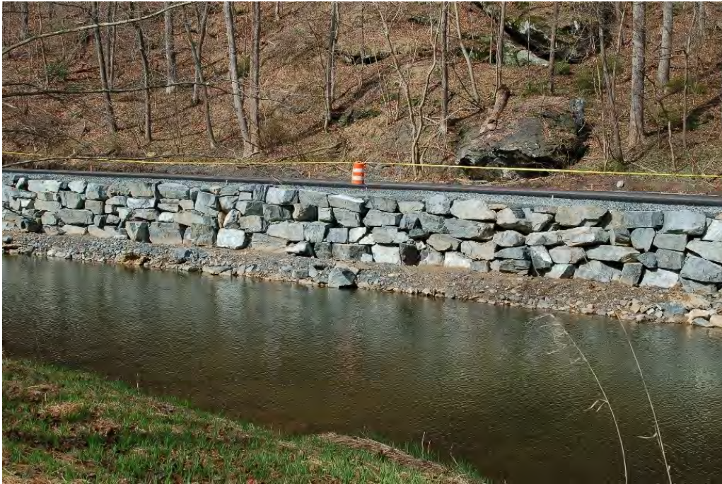
Photograph 1: Soil-filled riprap floodplain bench – installed in front of a boulder wall – during construction at Deer Creek, Harford County, MD. Source: JMT.
