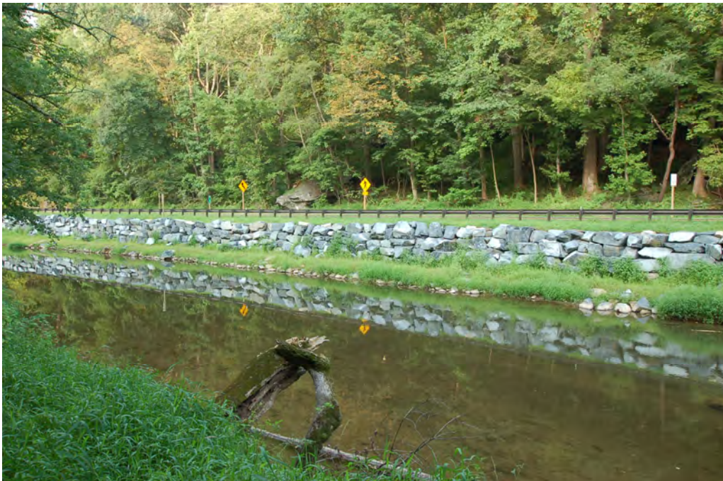
Photograph 2: Soil-filled riprap floodplain bench – installed in front of a boulder wall – following construction at Deer Creek, Harford County, MD. Source: JMT.
