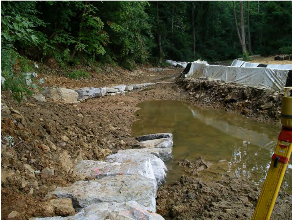
Photograph 1: Rock vane during construction at Middle Creek, Frederick County, MD. Source: JMT.
