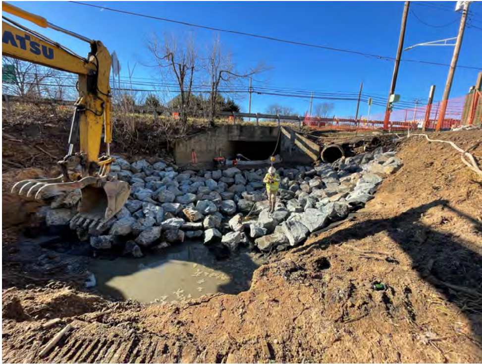
Photograph 1: Preformed scour hole during construction at UNT to Patapsco River, Baltimore County, MD. Source: JMT.
