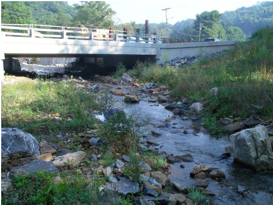
Photograph 2: Engineered habitat boulder placement following construction at Elklick Run, Allegany County, MD. Source: JMT.
