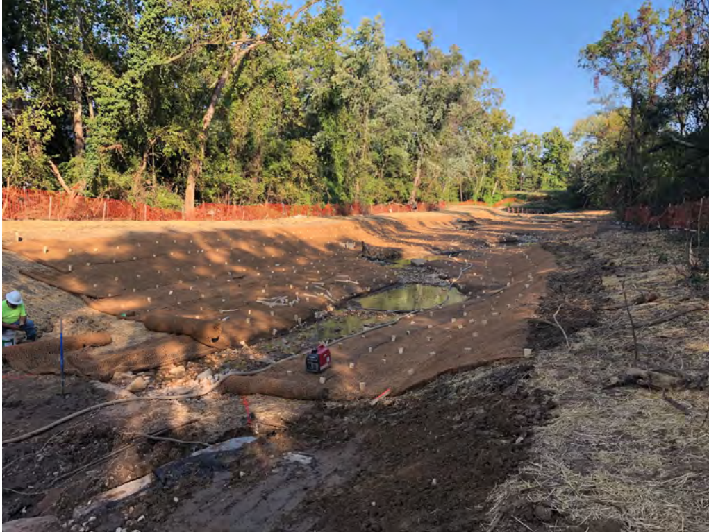
Photograph 1: Erosion control blanket during construction at UNT to Patapsco River, Baltimore County, MD. Source: JMT.
