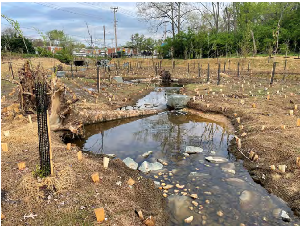
Photograph 2: Log vane-root wad following construction at UNT to Patapsco River, Baltimore County, MD. Source: JMT.
