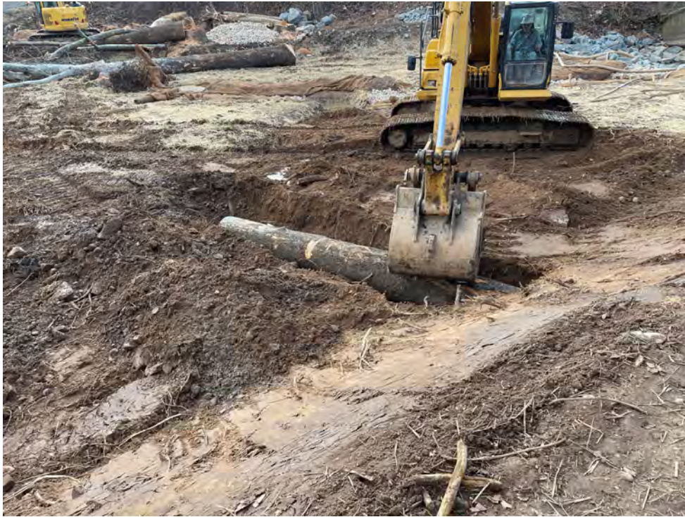
Photograph 1: Floodplain log sill during construction at UNT to Patapsco River, Baltimore County, MD. Source: JMT.
