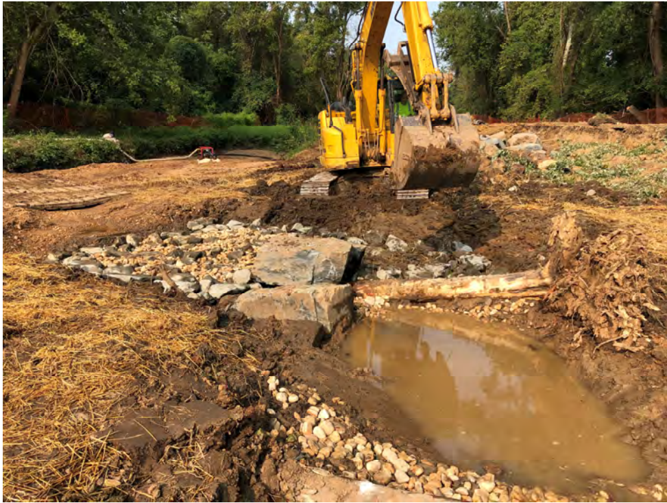
Photograph 1: Log vane-root wad during construction at UNT to Patapsco River, Baltimore County, MD. Source: JMT.
