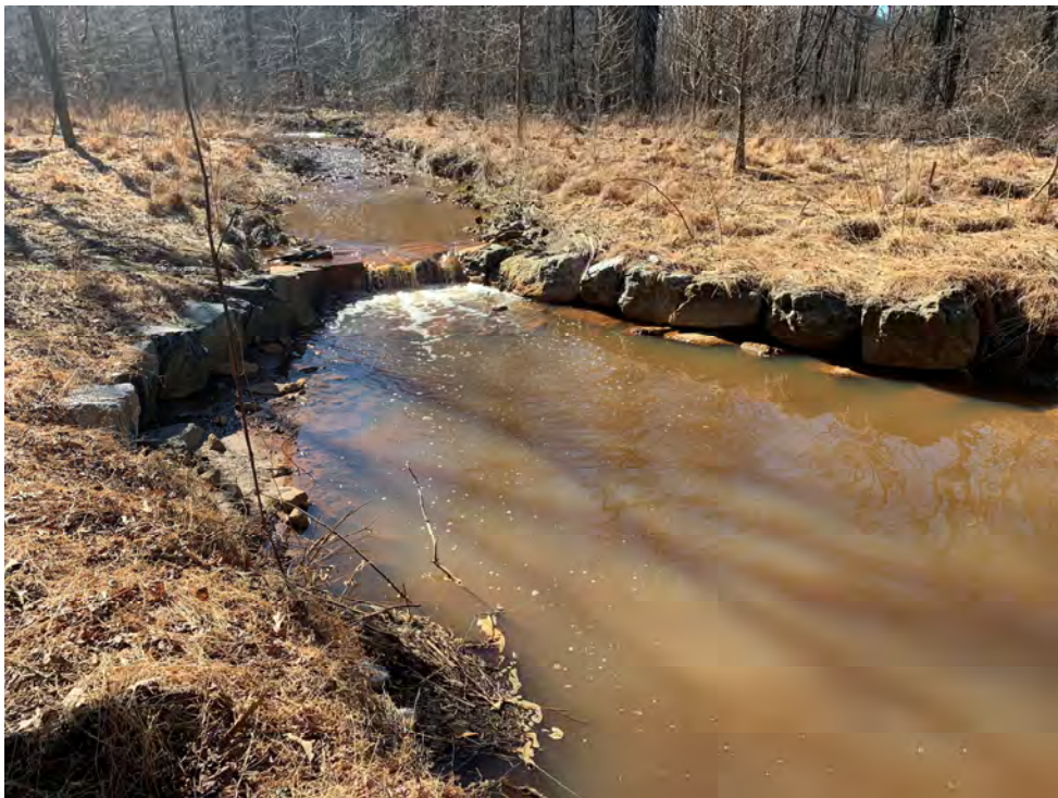
Photograph 2: Cross rock vane following construction at Kitten Branch, Anne Arundel County, MD. Source: JMT.
