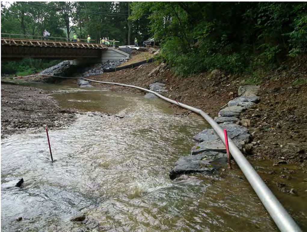
Photograph 2: Rock Vane following construction at Middle Creek, Frederick County, MD. Source: JMT.
