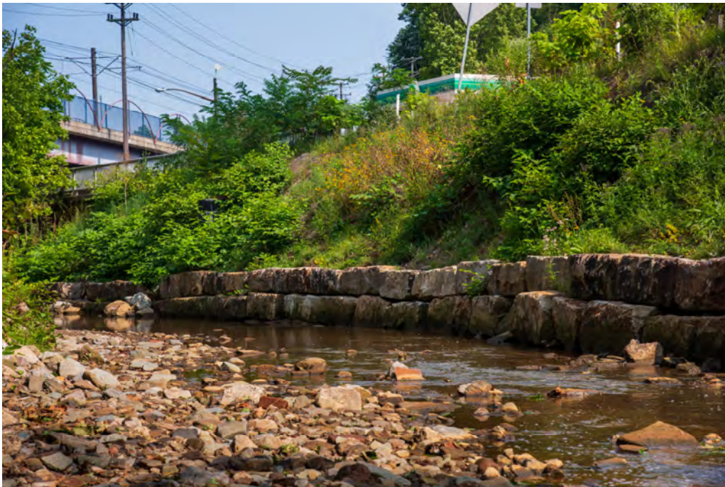
Photograph 2: Boulder toe revetment following construction at Saw Mill Run, Allegheny County, PA. Source: JMT.
