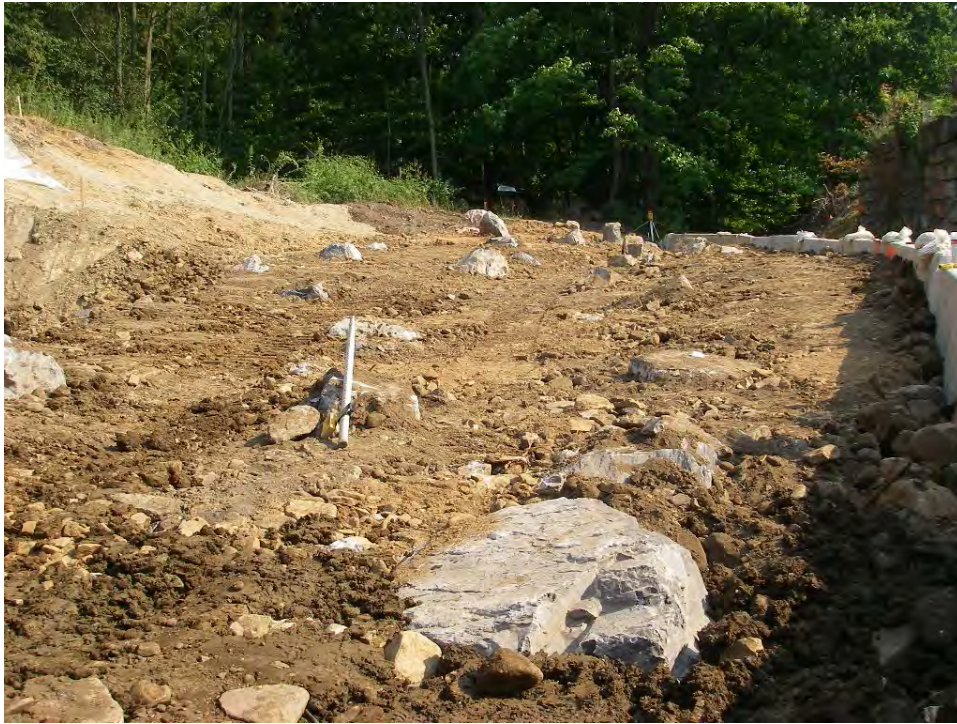
Photograph 1: Engineered habitat boulder placement during construction at Elklick Run, Allegany County, MD. Source: JMT.
