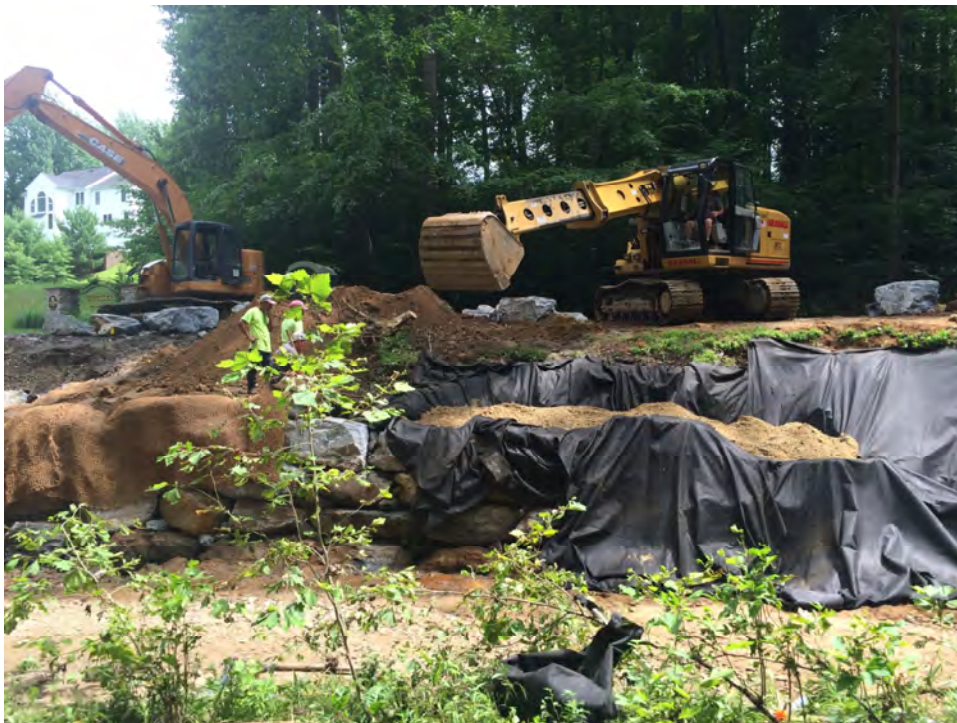
Photograph 2: Boulder wall during construction at UNT Middle Patuxent River, Howard County, MD; showing installation of filter stone backfill to be wrapped in non-woven geotextile. Source: JMT.
