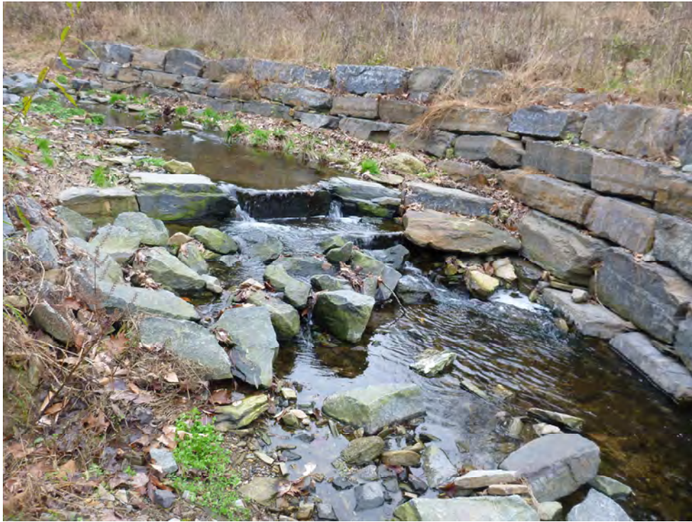
Photograph 1: Rock step pool with boulder toe revetment following construction at West Branch Indian Creek, Philadelphia, PA. Source: PWD.
