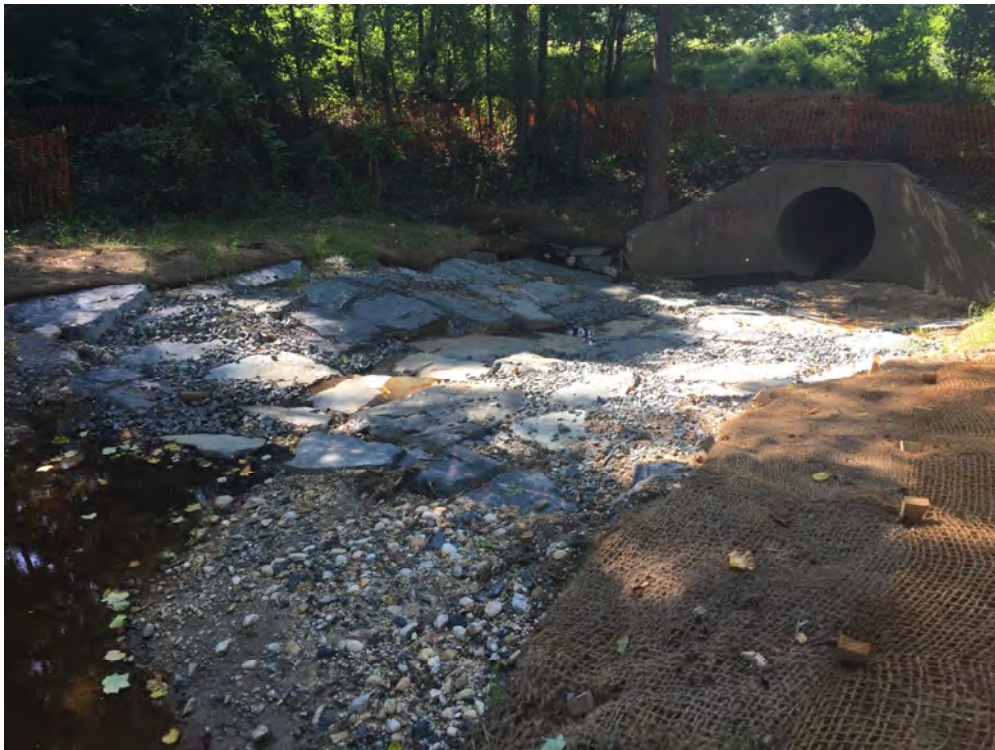
Photograph 2: Boulder cascade following construction at White Marsh Run Tributary, Baltimore County, MD. Source: JMT.
