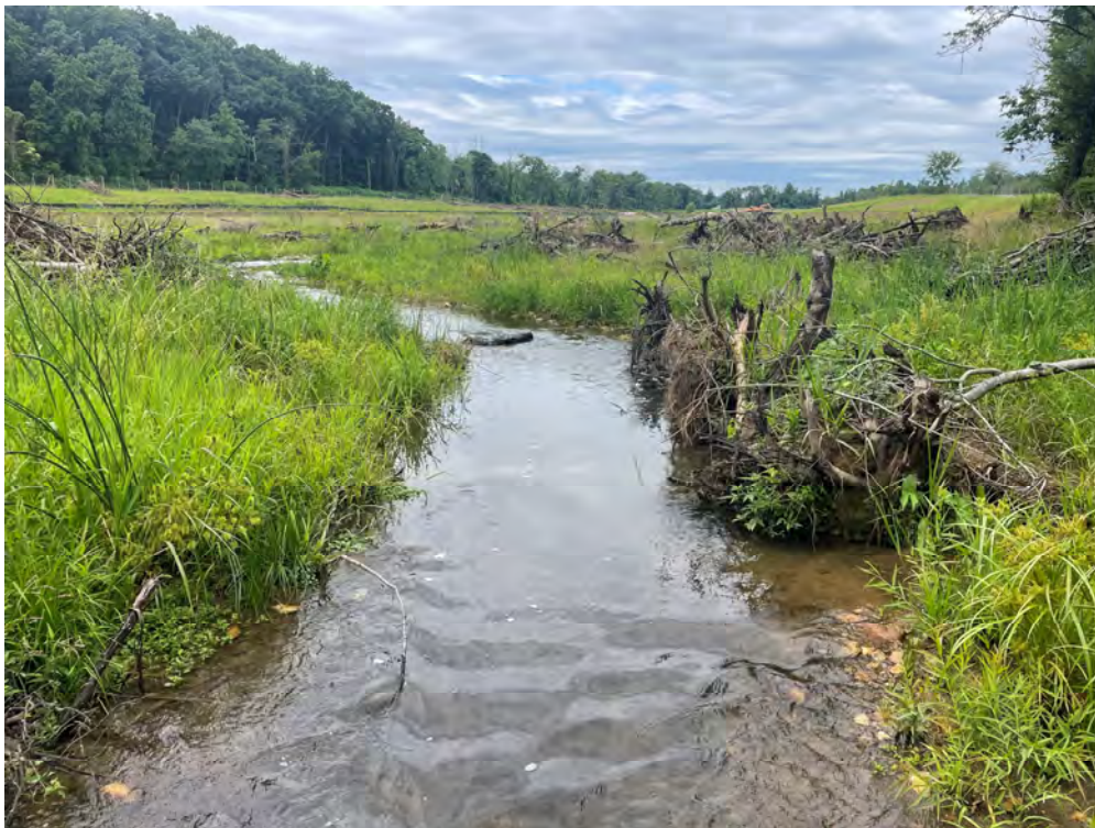
Photograph 2: Toe wood following construction at Jones Falls, Baltimore County, MD. Source: JMT.
