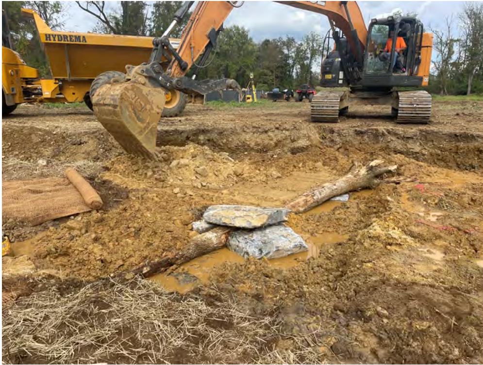
Photograph 1: Log vane during construction at UNT to Jones Falls, Baltimore County, MD. Source: JMT.
