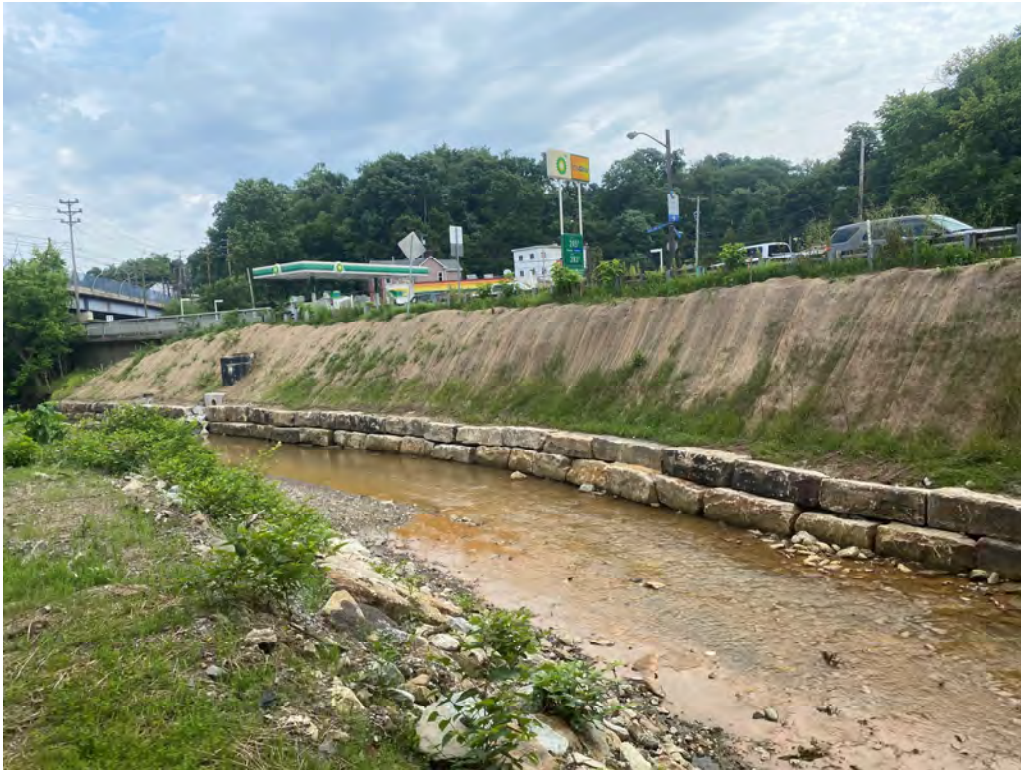
Photograph 1: Boulder toe revetment during construction at Saw Mill Run, Allegheny County, PA. Source: JMT.
