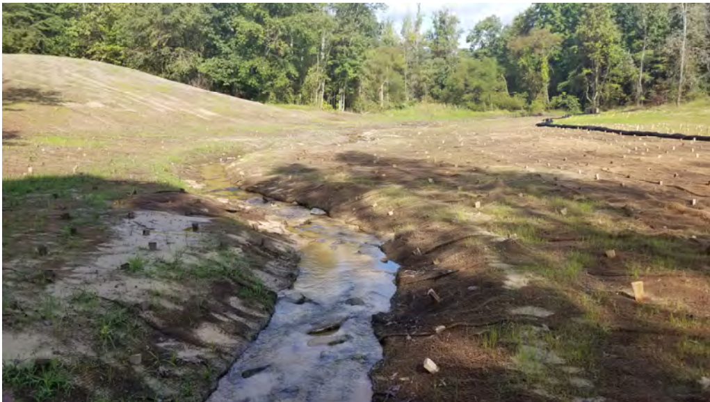
Photograph 2: Erosion control blanket following construction at Bear Branch, Anne Arundel County, MD. Source: JMT.
