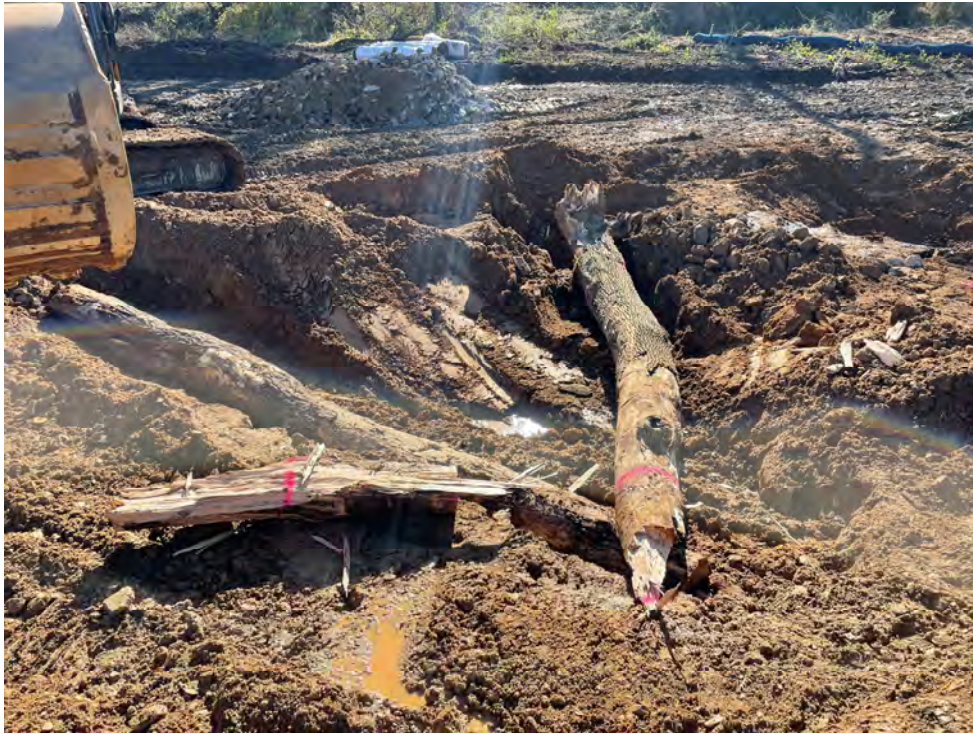
Photograph 1: Rock and roll logs during construction at UNT to Jones Falls, Baltimore County, MD. Source: JMT.
