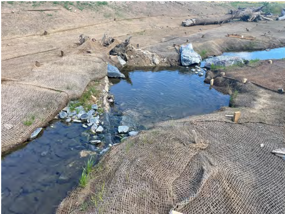
Photograph 2: Log vane following construction at UNT to Jones Falls, Baltimore County, MD. Source: JMT.
