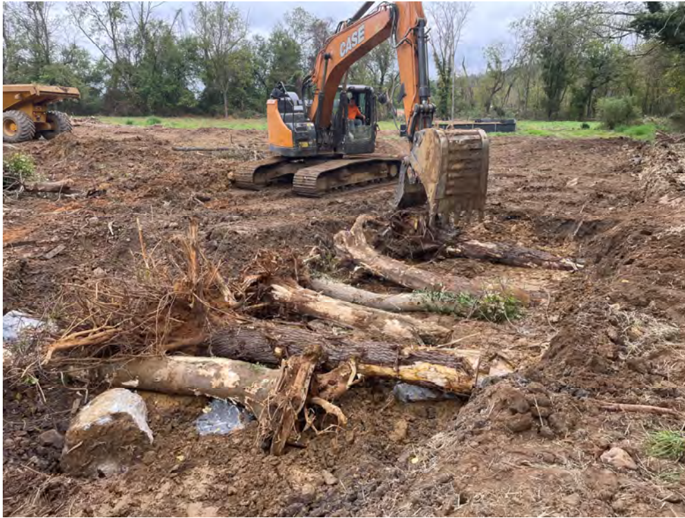
Photograph 1: Toe wood during construction at UNT to Jones Falls, Baltimore County, MD. Source: JMT.
