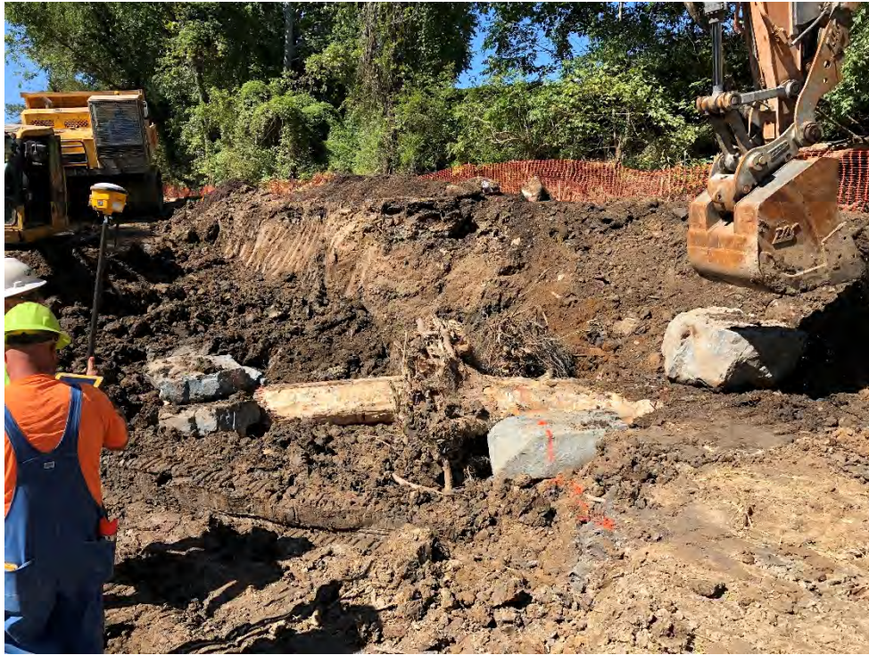
Photograph 1: Root wad during construction at UNT to Patapsco River, Baltimore County, MD. Source: JMT.
