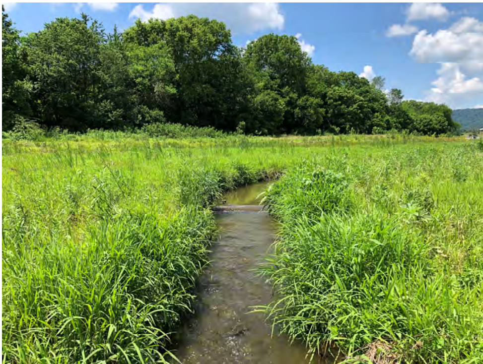
Photograph 2: In-stream log sill following construction at Little Catoctin Creek, Frederick County, MD. Source: JMT.
