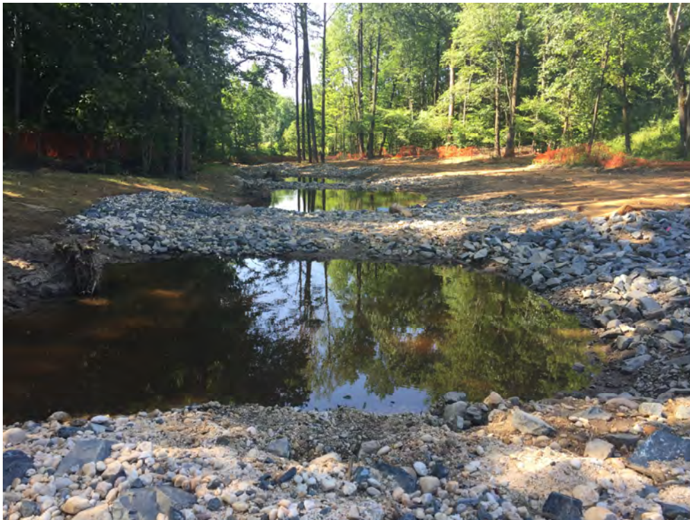
Photograph 2: Regenerative step pool storm conveyance following construction at White Marsh Run Tributary, Baltimore County, MD. Source: JMT.
