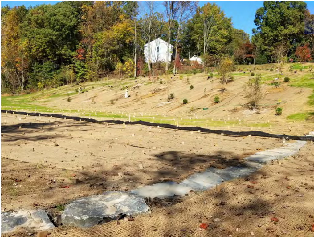
Photograph 1: Rock sill during construction at Bear Branch, Anne Arundel County, MD. Source: JMT.
