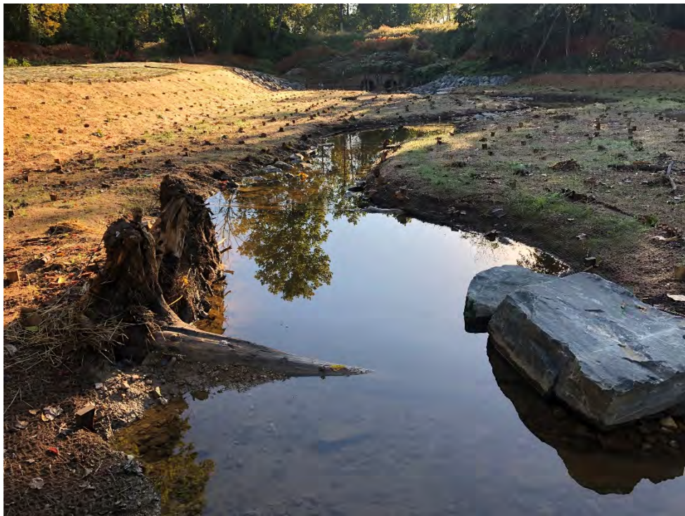
Photograph 2: Root wad following construction at UNT to Patapsco River, Baltimore County, MD. Source: JMT.
