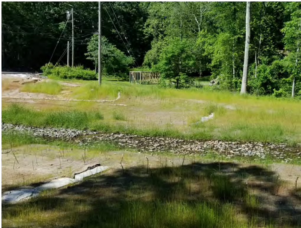
Photograph 2: Rock sill following construction at Bear Branch, Anne Arundel County, MD. Source: JMT.
