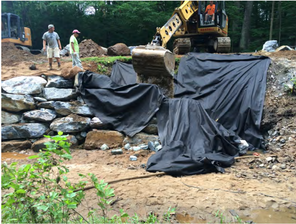
Photograph 1: Boulder wall during construction at UNT Middle Patuxent River, Howard County, MD; showing preparation of non-woven geotextile and beginning of filter stone backfill installation.
