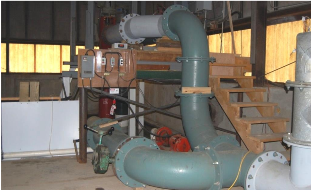
Figure 9 Photograph Showing Laboratory Pumps
