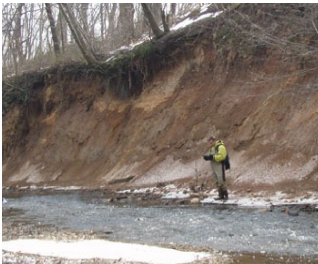
Figure 1. Eroded stream bank at Poquessing Creek
