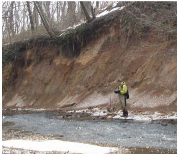
Figure 1. Eroded stream bank at Poquessing Creek
