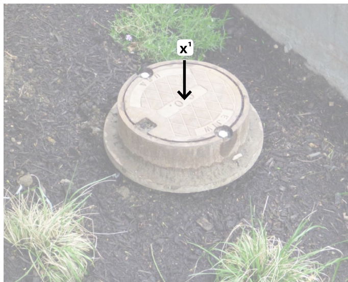
Rim elevation: center point at top of cleanout cover.
