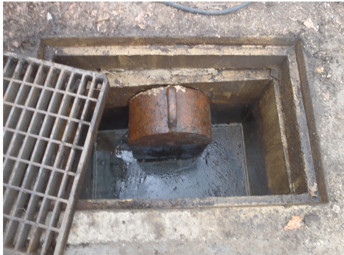
Inlet hood: view from above.
