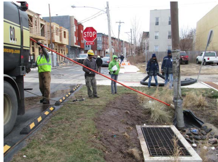
Shissler Recreation Center - Crews performing routine subsurface maintenance on a rain garden.
