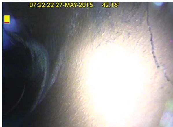
Figure 3-13. Circumferential Fracture, a Break Line that is Visibly Open and a Gap Can be Seen. The Sections of Pipe Wall are Still in Place and Cannot Move.
