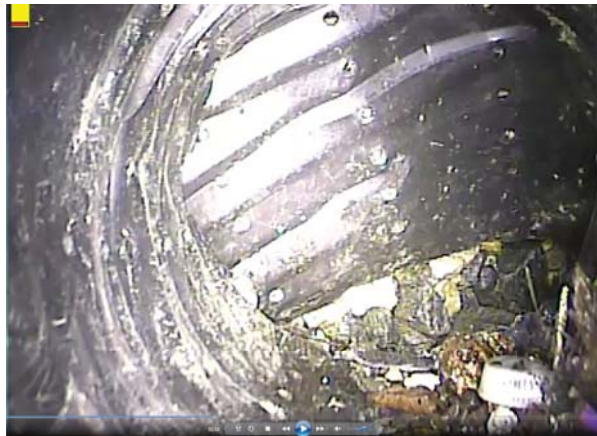
Figure 3-17. Collapse, Deformation so Great that there has been a Complete Loss of the Structural Integrity of the Pipe with More than 40% of Cross-sectional Area Lost.
