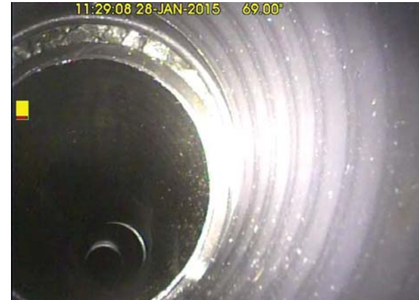
Figure 3-18. Offset Joint, a Defective Displacement of at Least One Pipe Thickness at a Joint.
