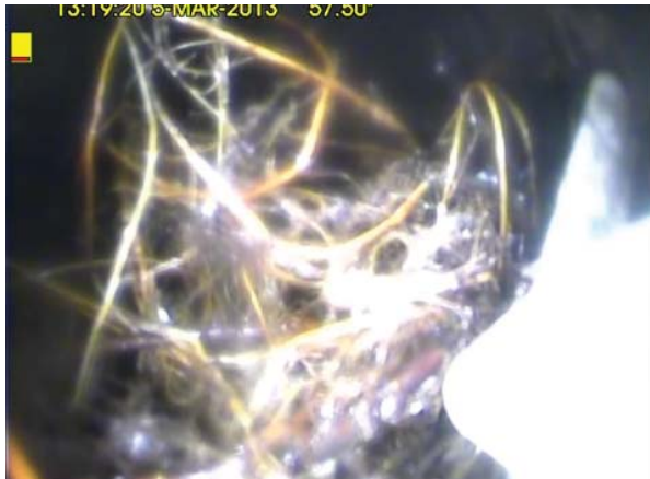
Figure 3-23. Root - Ball: Roots that have Formed a Mass, Typically in the Form of a Ball, and have the Potential to Severely Restrict the Flow. The Cross-sectional Area is Greater than 50%.
