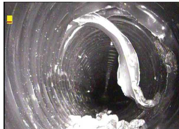
Figure 3-15. Hole, a Defect Where Pipe Material is Completely Dislodged from Pipe Wall and the Surrounding Media is Exposed.
