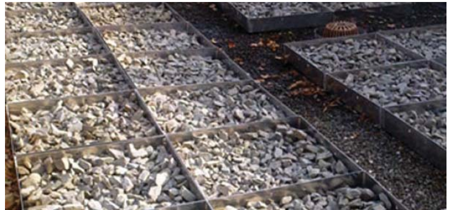
Figure 1-29. Examples of Blue Roofs in New York City (Image credit: Gowanus Canal Watershed, Hazen and Sawyer)
