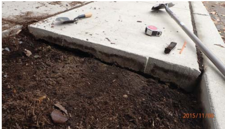
Figure 2-5. Example of Settling in a Tree Pit
