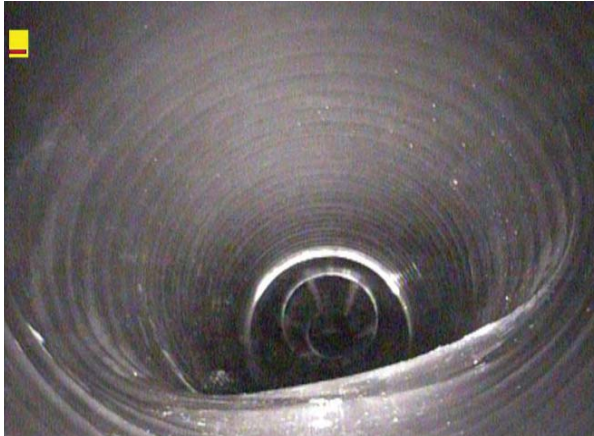
Figure 3-16. Deformation, Pipe Damage Where the Original Cross-section or Geometry of the Pipe has Noticeably Changed.
