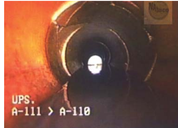
Figure 3-14. Break, a Defect Where Pieces are Noticeably Displaced and Have Moved from Original Position at Least \frac{1}{2} the Thickness of the Pipe.
