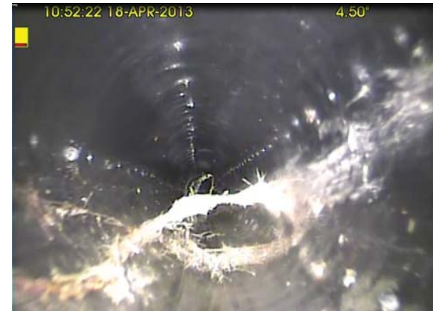
Figure 3-22. Roots - Medium: Roots that have Formed a Mass and Restrict the Flow of Water. Cross-sectional Area Lost is Greater than or Equal to 5% up to or Less than or Equal to 50% (5-50%).
