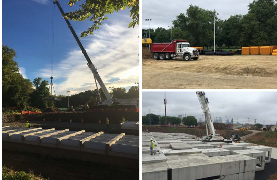
Figure 47: Examples of GSI sewers during construction. From left to right, top to bottom: Ferko Playground, Wissinoming Park, Lanier Playground.
