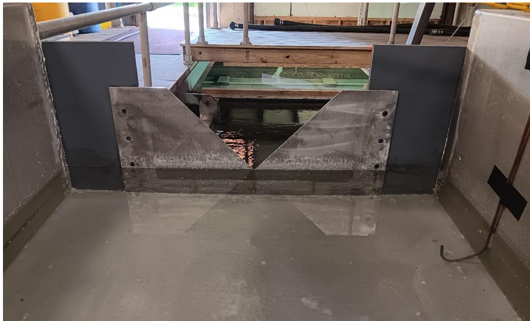
Figure 7 Effluent Channel V-notch Weir
