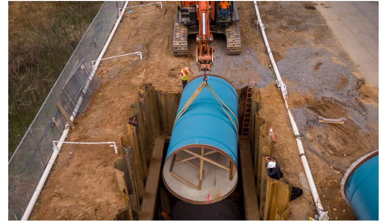
Example of a large transmission main
