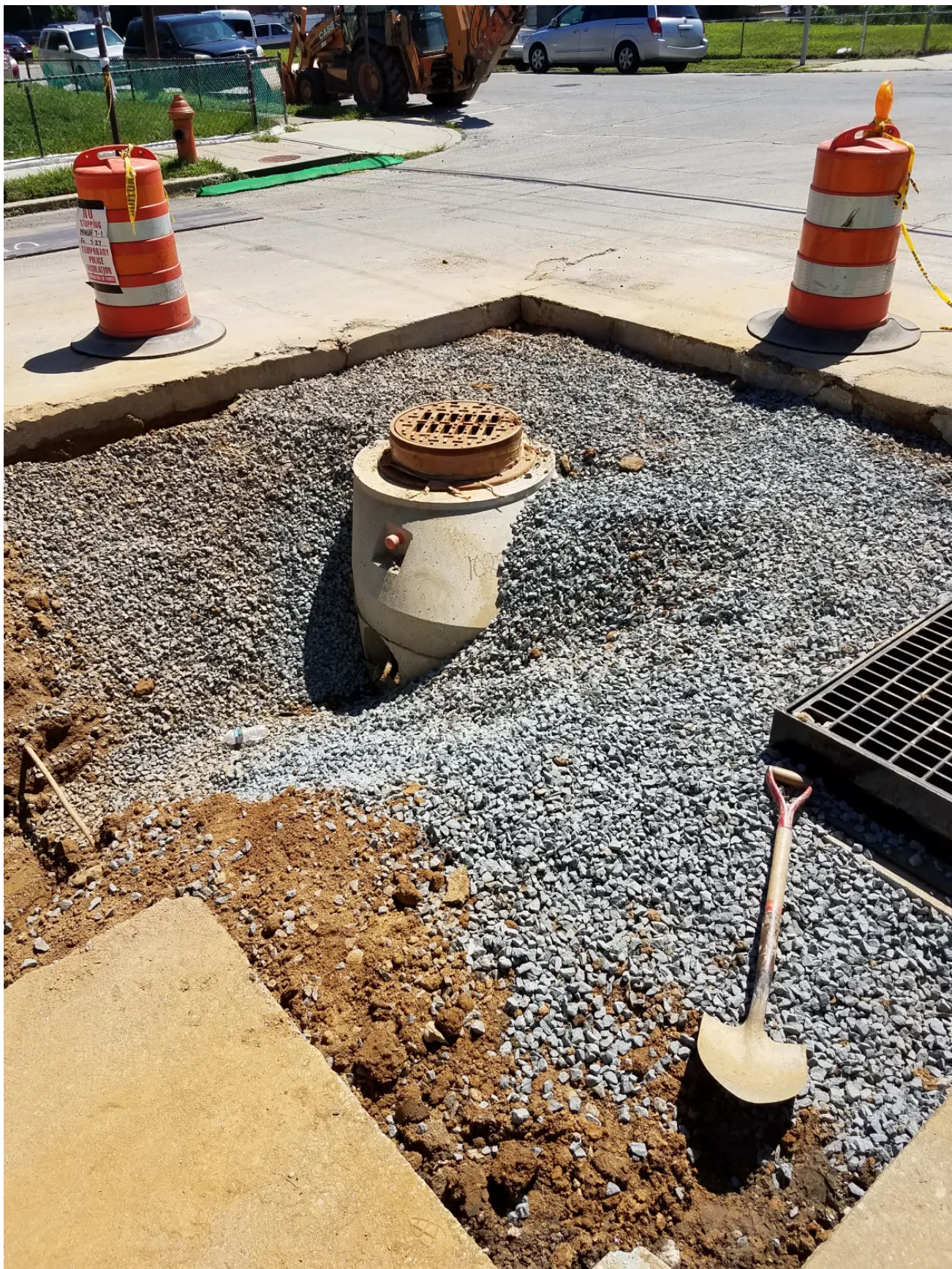
An example of a precast concrete drainage well in Philadelphia
