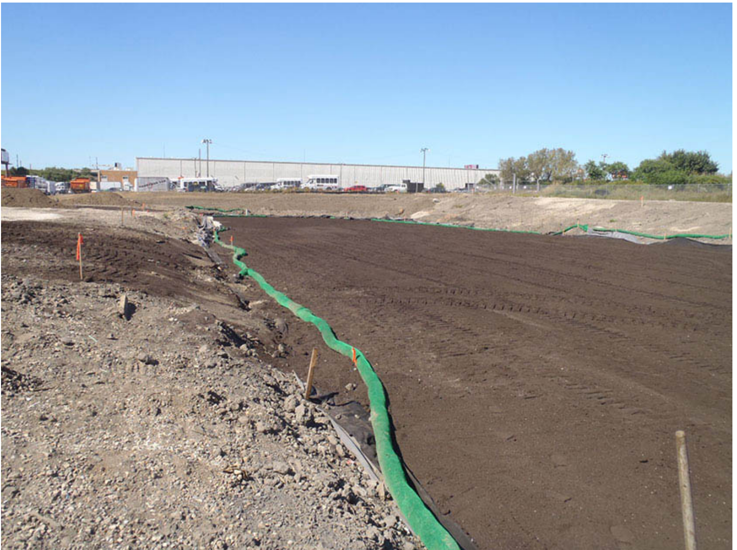
An example of a wet basin installation in Philadelphia
