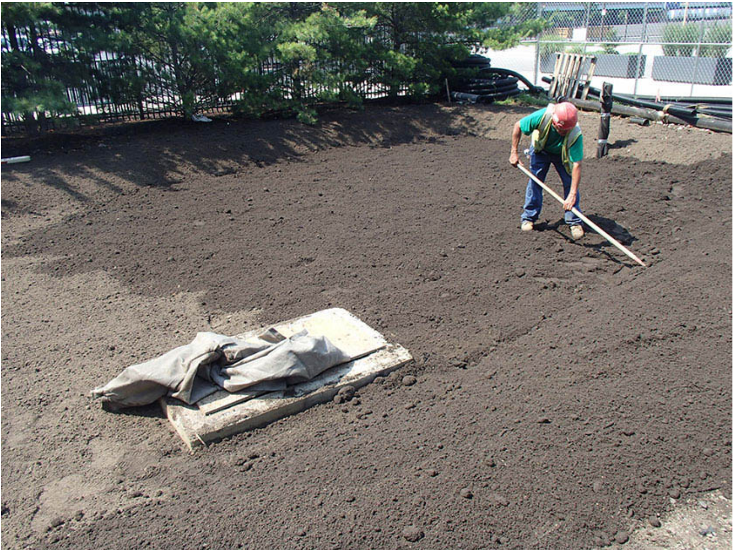
An example of a bioinfiltration basin installation in Philadelphia
