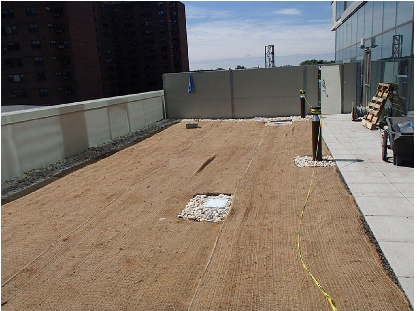
An example of a green roof installation in Philadelphia
