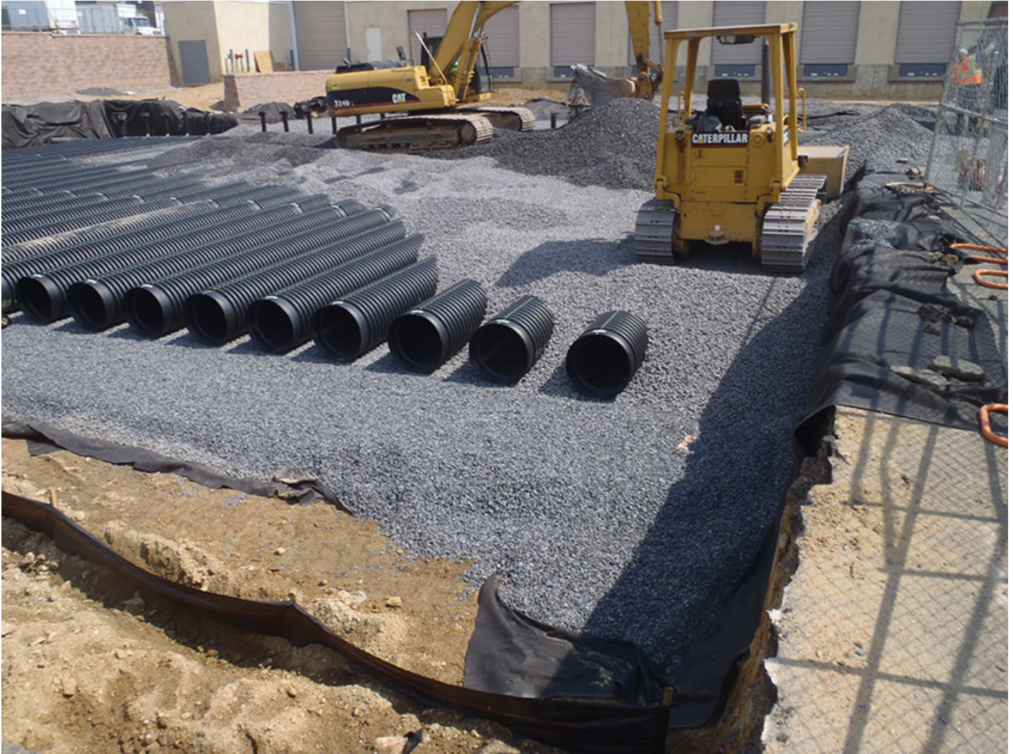
An example of a subsurface infiltration basin installation in Philadelphia
