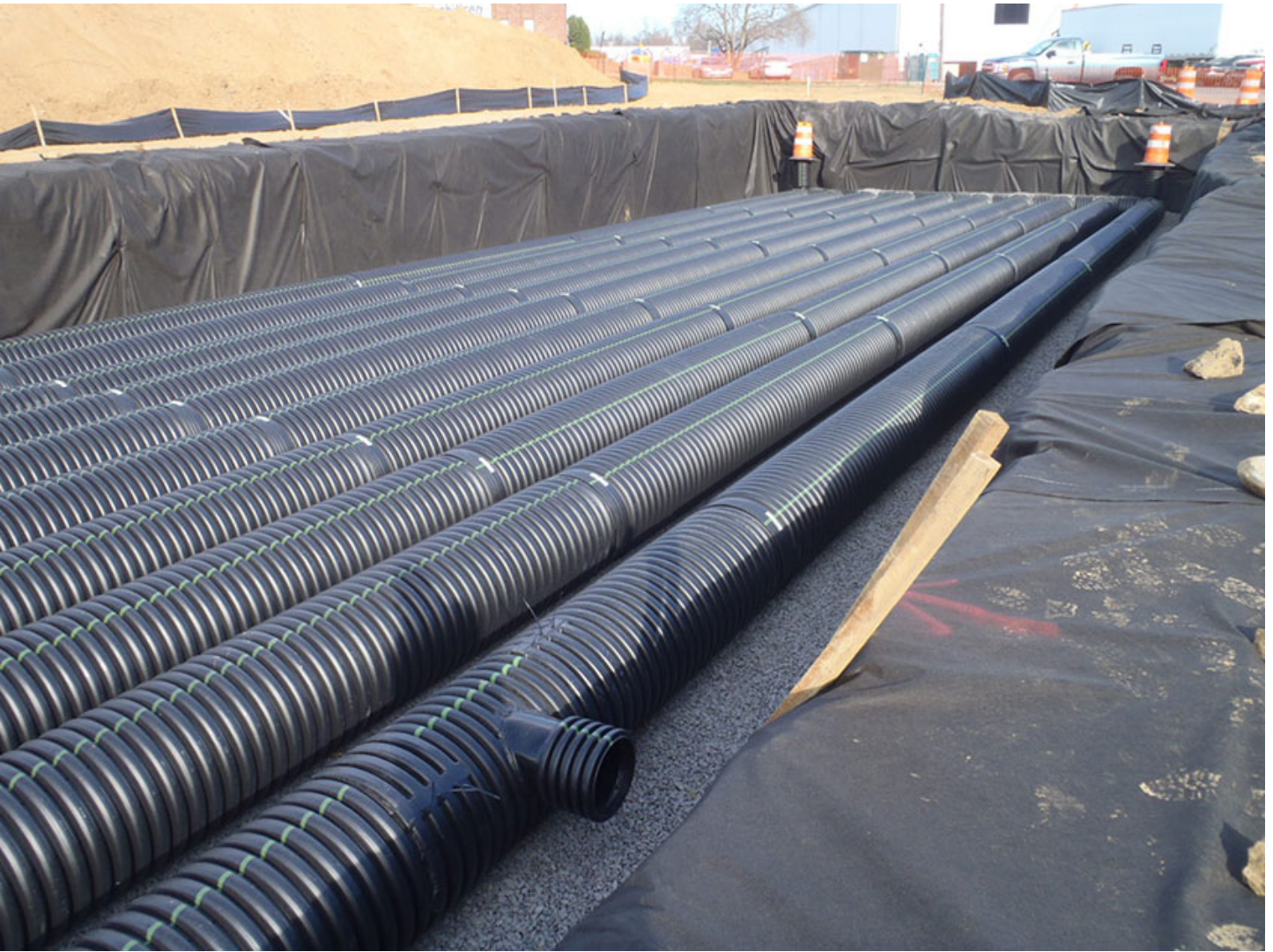
An example of a subsurface infiltration basin in Philadelphia
