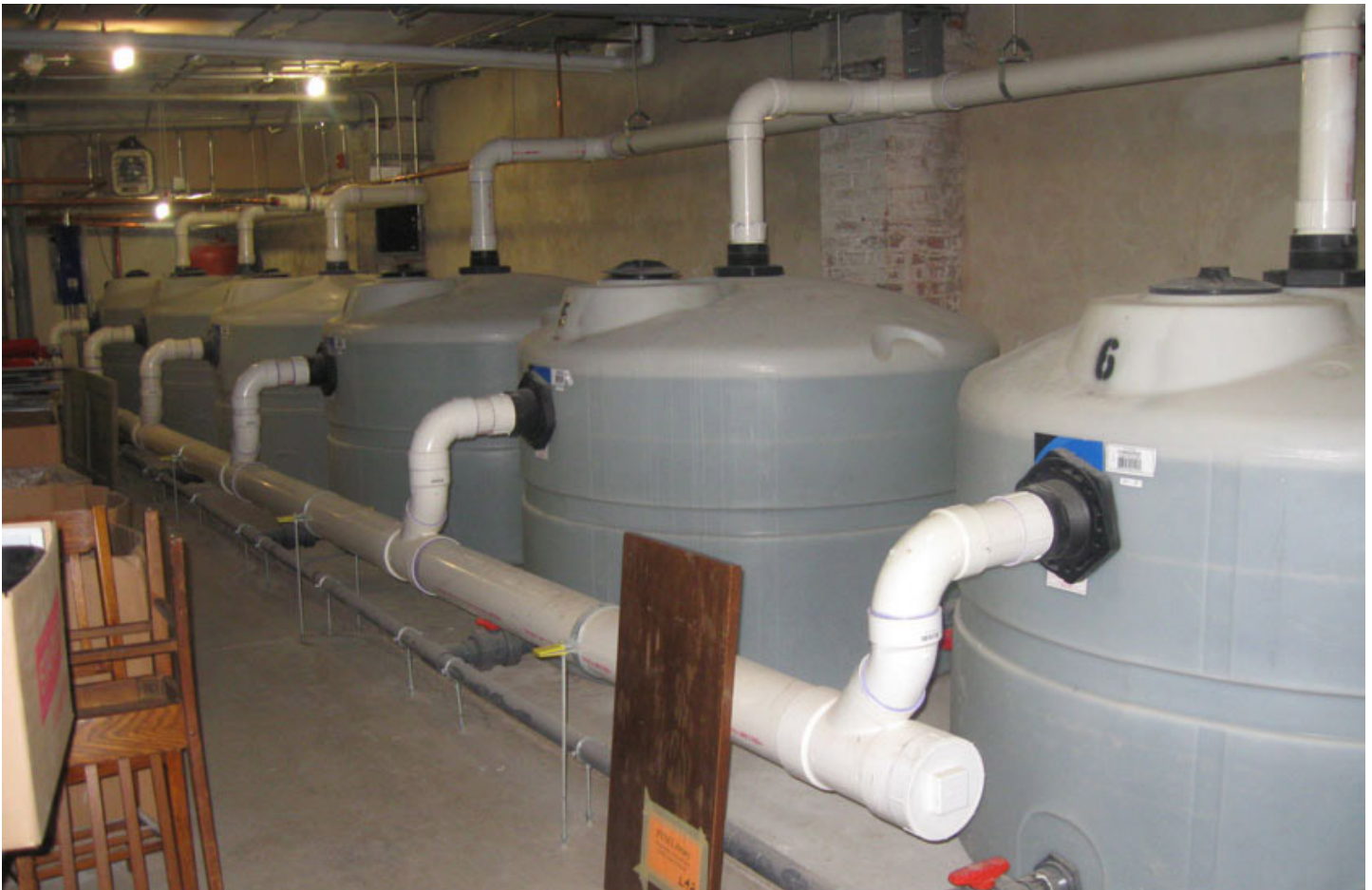
An example of a subsurface cistern in Philadelphia
