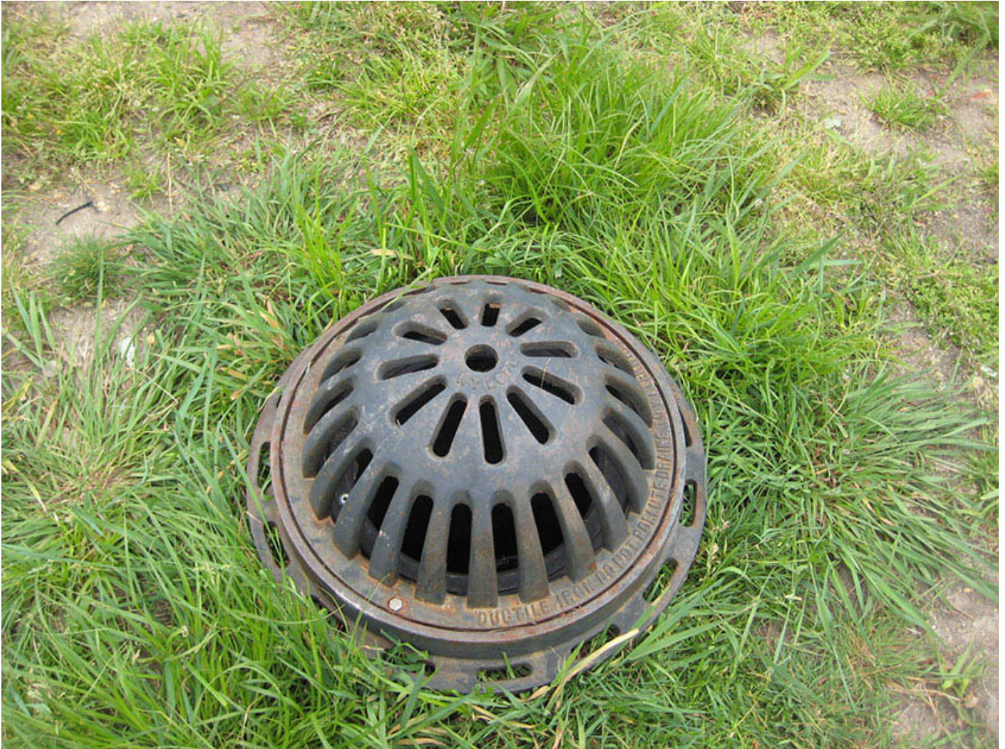
An example of a domed riser pipe in Philadelphia
