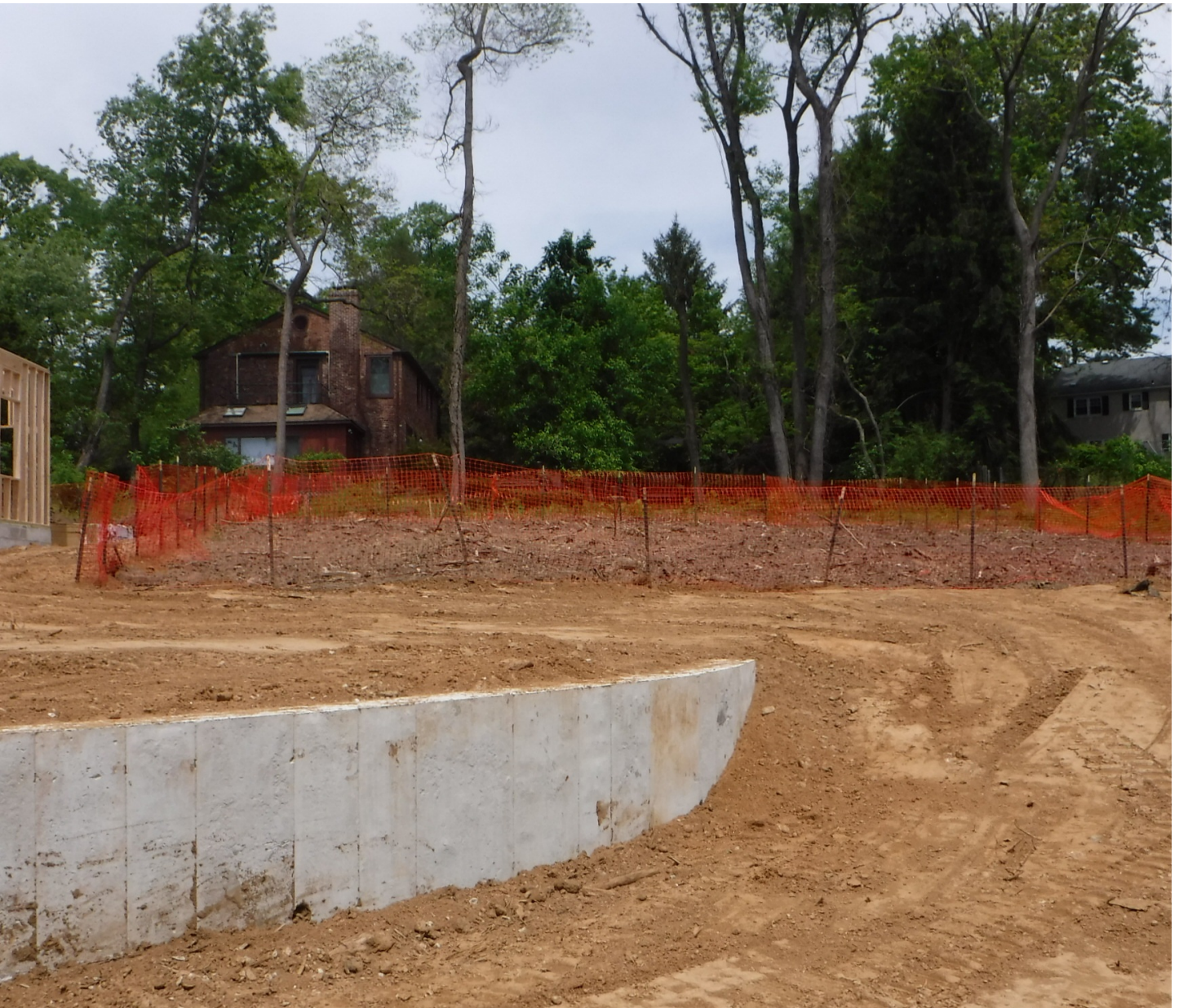
An example of infiltration area marking to avoid compaction during construction in Philadelphia
