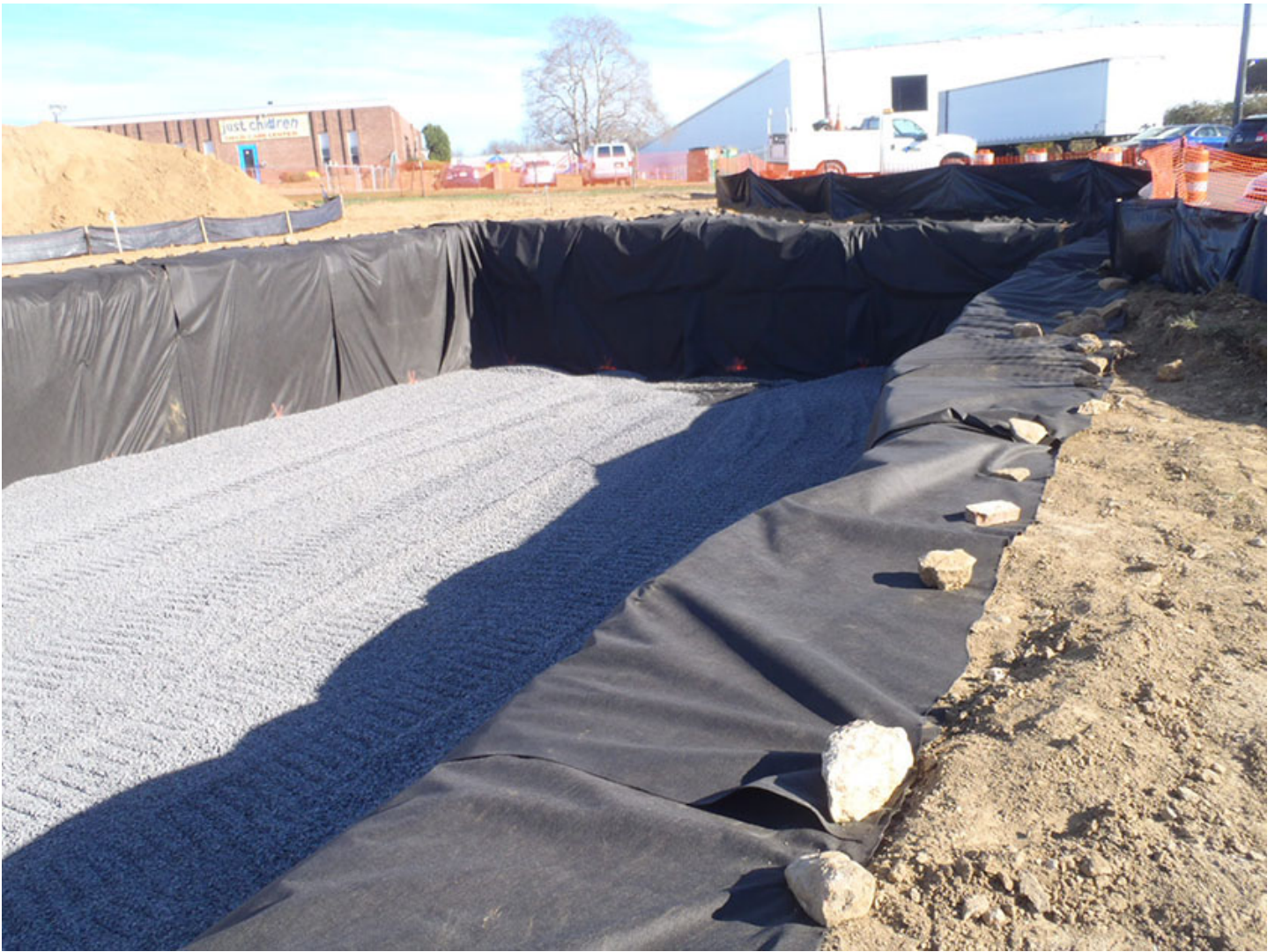
An example of a subsurface detention basin installation in Philadelphia
