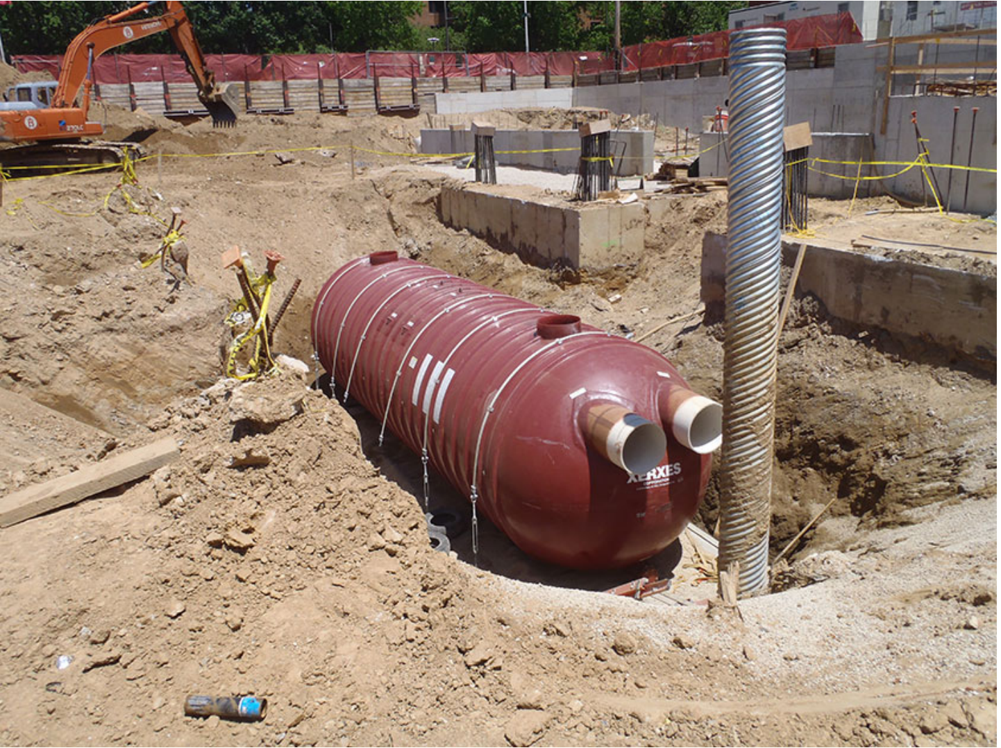
An example of a subsurface cistern installation in Philadelphia
