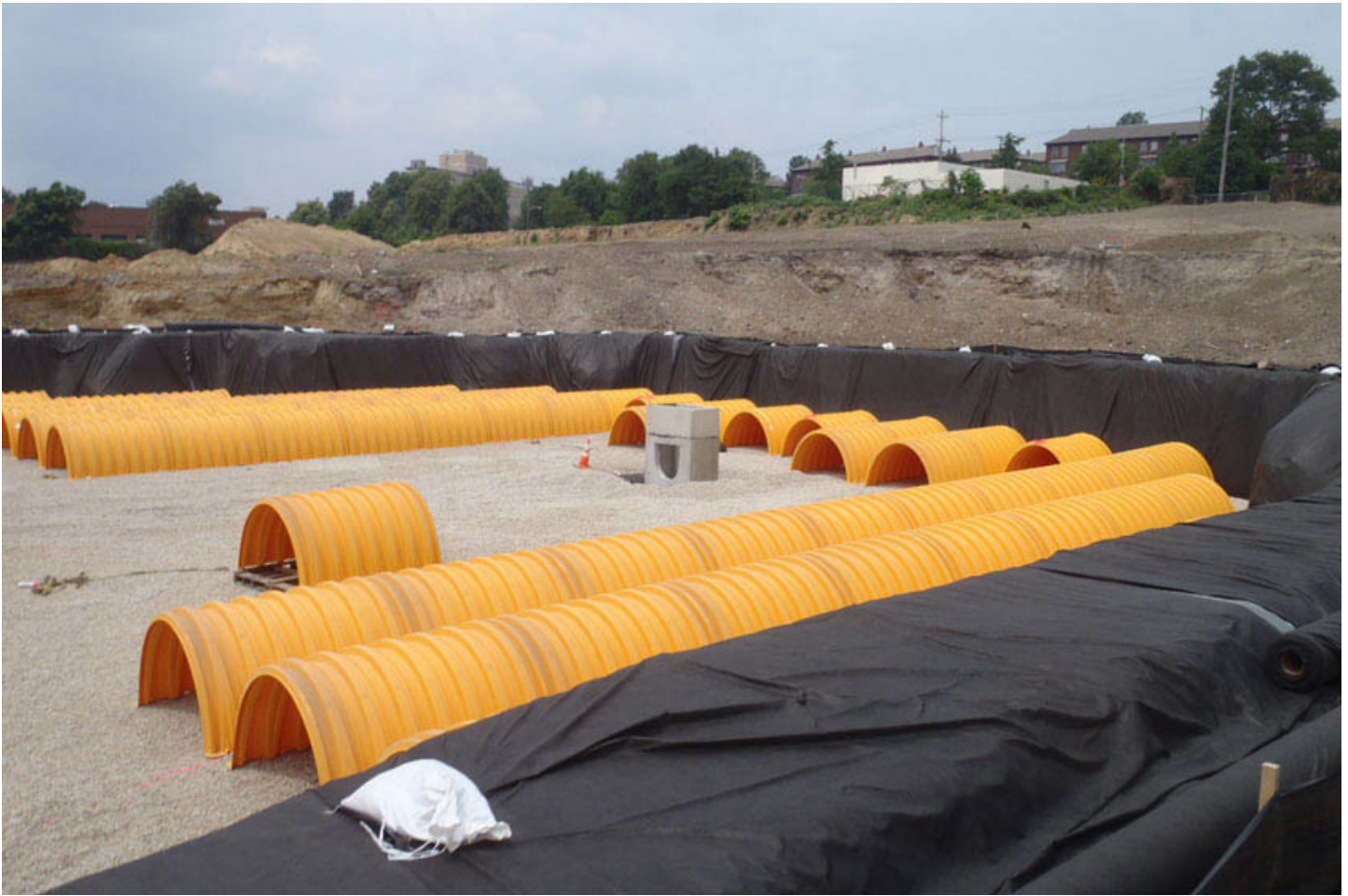
An example of a subsurface detention basin in Philadelphia
