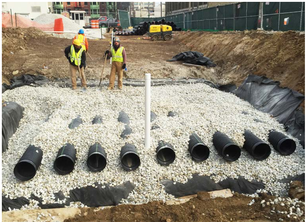
During construction, construction crews install layers of soil, rock, and drains that exist beneath the parking lot to divert sewer overflows away from waterways. Photo © INTECH Construction
