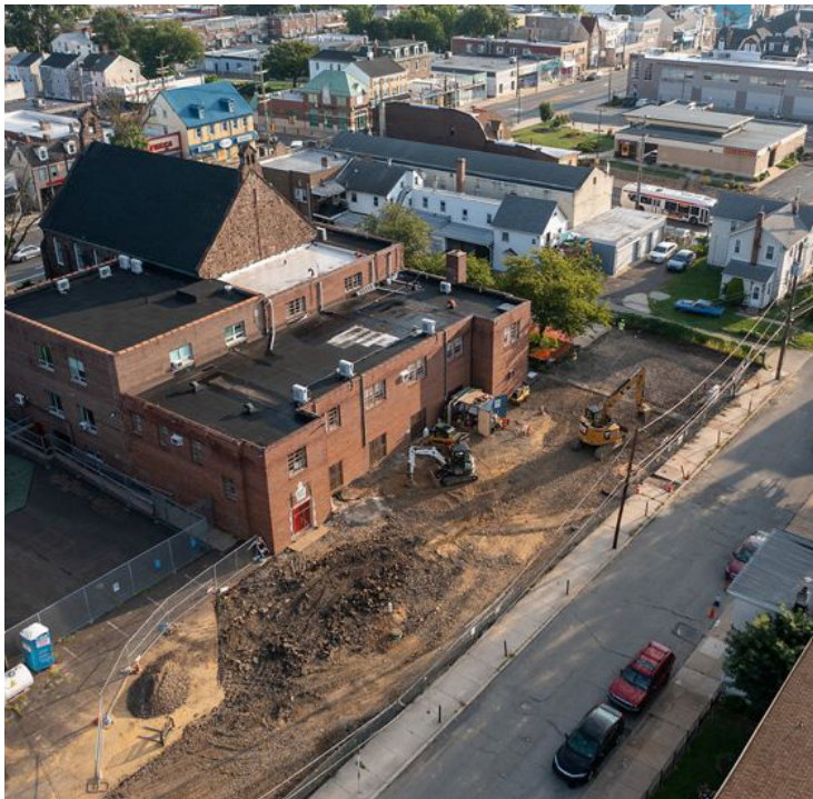
In mid-2021, crews work on repaving the rear parking area after installing a subsurface basin. Photo © Oak Leaf Media
